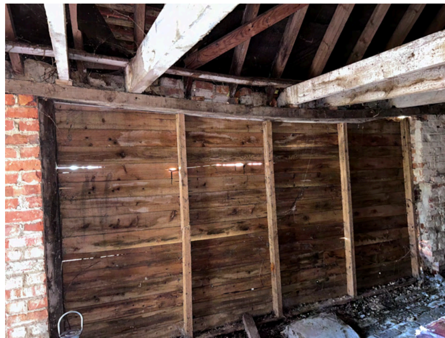
Fig. 13, Existing roof structure, significantly reduced support for part of the roof, structure sagging.
