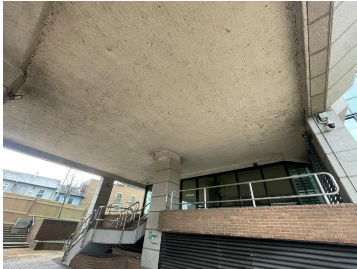
Photo 5: undercroft area, subject to infilling
