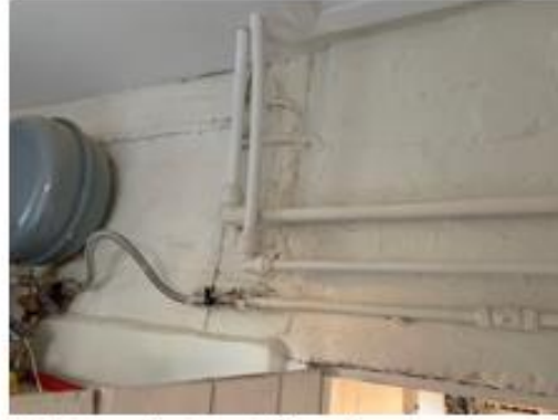
Fig 5a Internal pipework (historic north east wall, lobby side)
