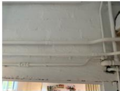
Fig 3a Internal pipework (historic north east wall, lobby side)
