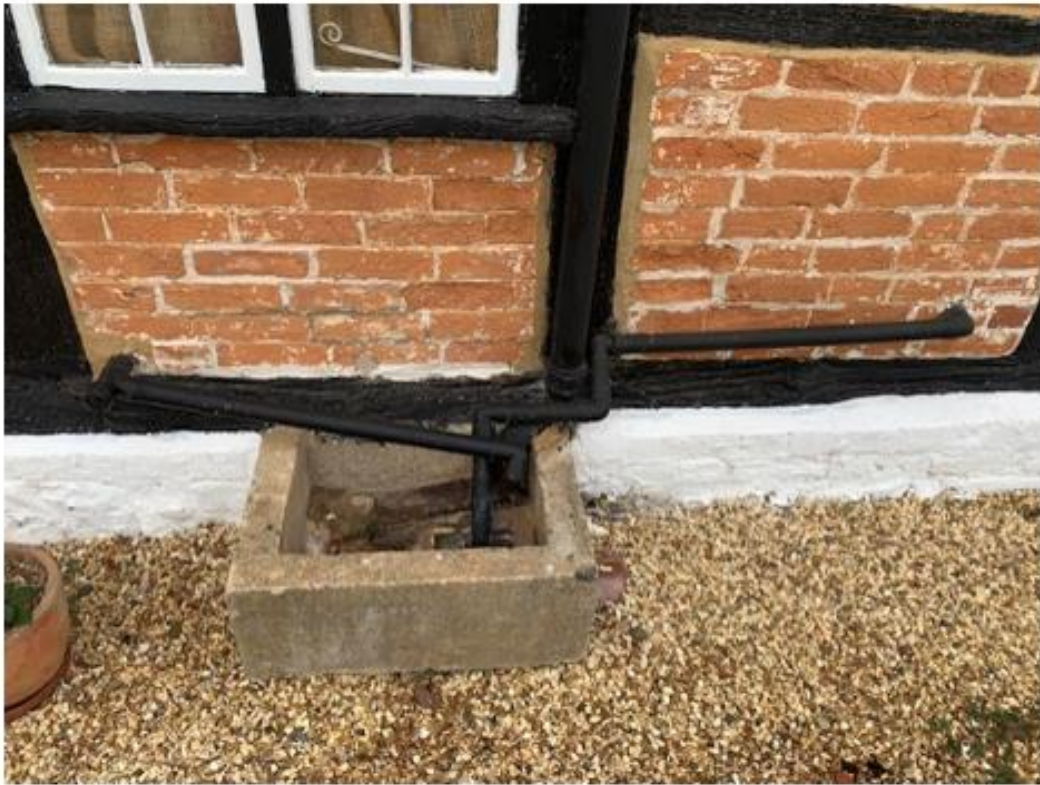
Fig 1a. External sink and washing machine outlet gulley (historic south east wall)
