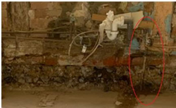
Fig. 8a. Mains inlet pipe (circled red), sink trap and waste, hot and cold water supply. These were exposed when the sand and cement internal render was removed. Signs of historic leakage and damp can be seen at the base of the pipe.
