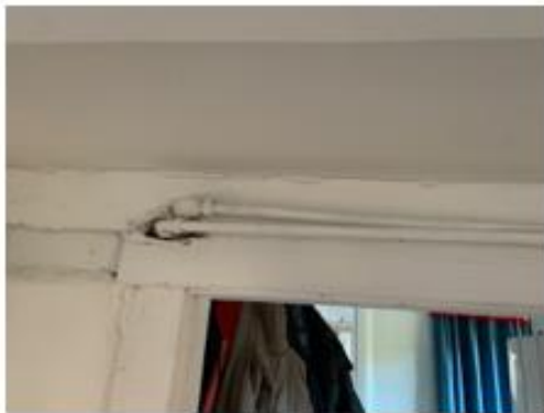
Fig 2a Internal pipework in kitchen (historic north east wall, kitchen side).
