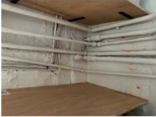
Fig 4a Internal pipework (historic north east wall, lobby side).
