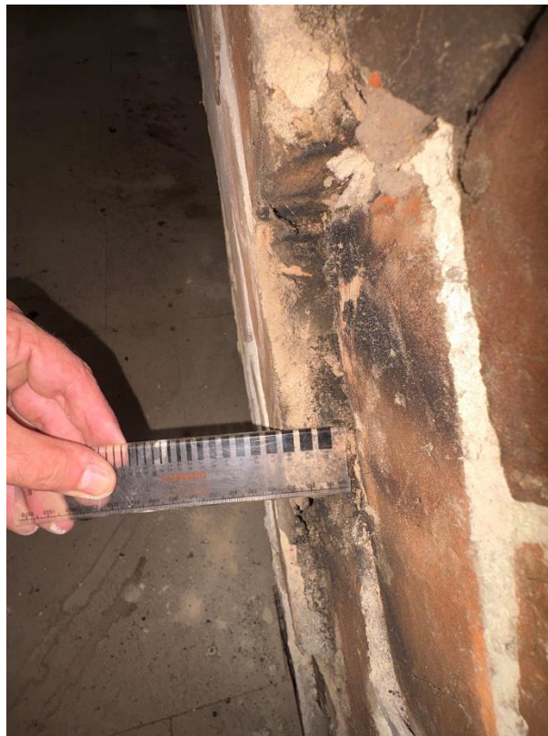
Figure 8. Chimney stack – 7 Victoria Street – lateral movement.
