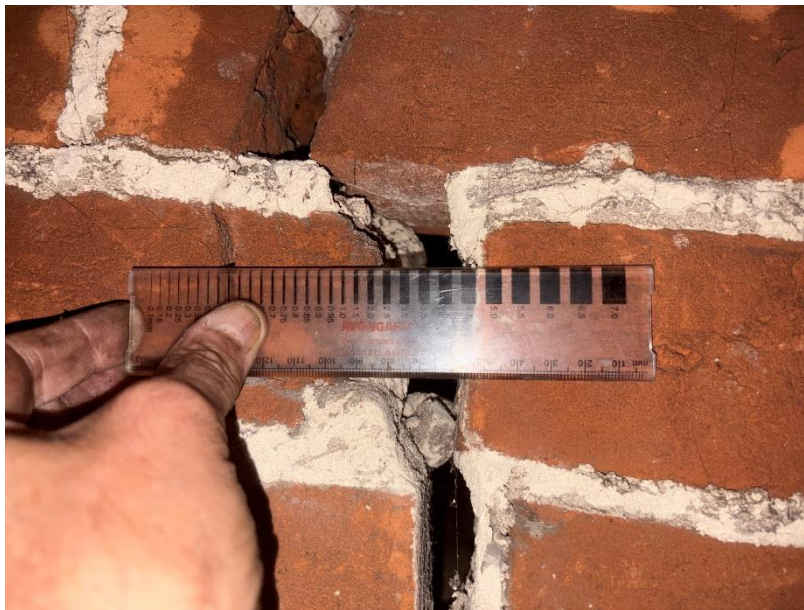
Figure 5. Cracking to brick panel beneath arched stack.
