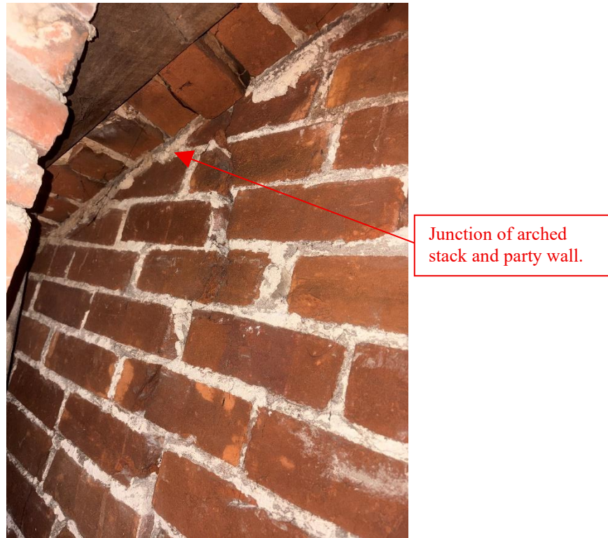
Figure 4. Junction of stack and party wall + Cracking to brick panel beneath arched stack.
