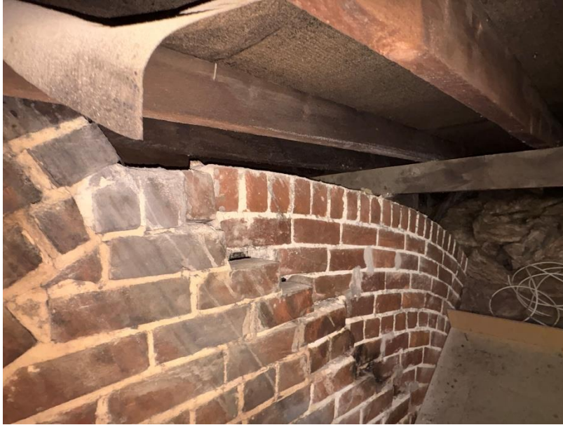
Figure 7. Chimney stack – 7 Victoria Street – lateral movement.
