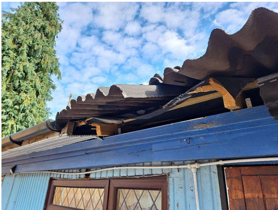
Fig 2. Detail showcasing the large gap in the soffit and fascia boarding along the western aspect.
