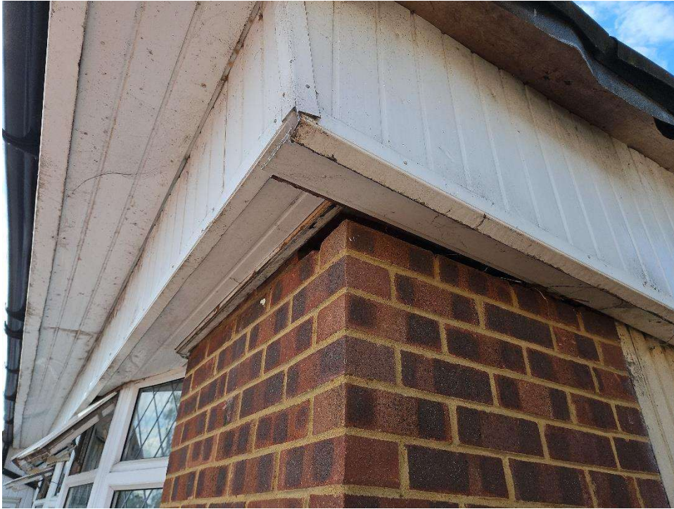
Fig 3. View of a prominent gap between the external boarding and brick wall on the north-eastern corner of the site.
