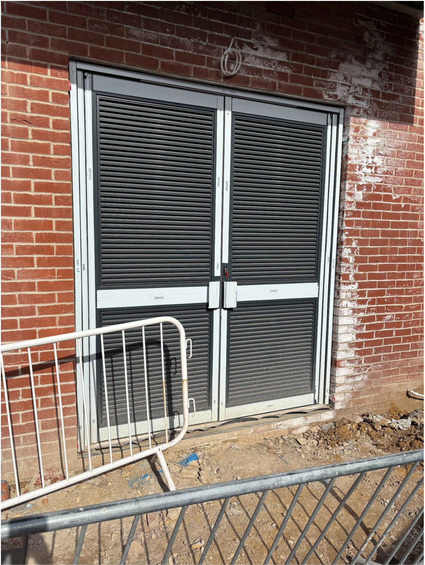
Photo of Binstore Door
