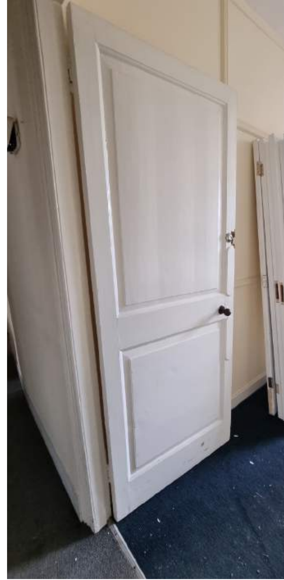
Door to be closed off as per approved application.
