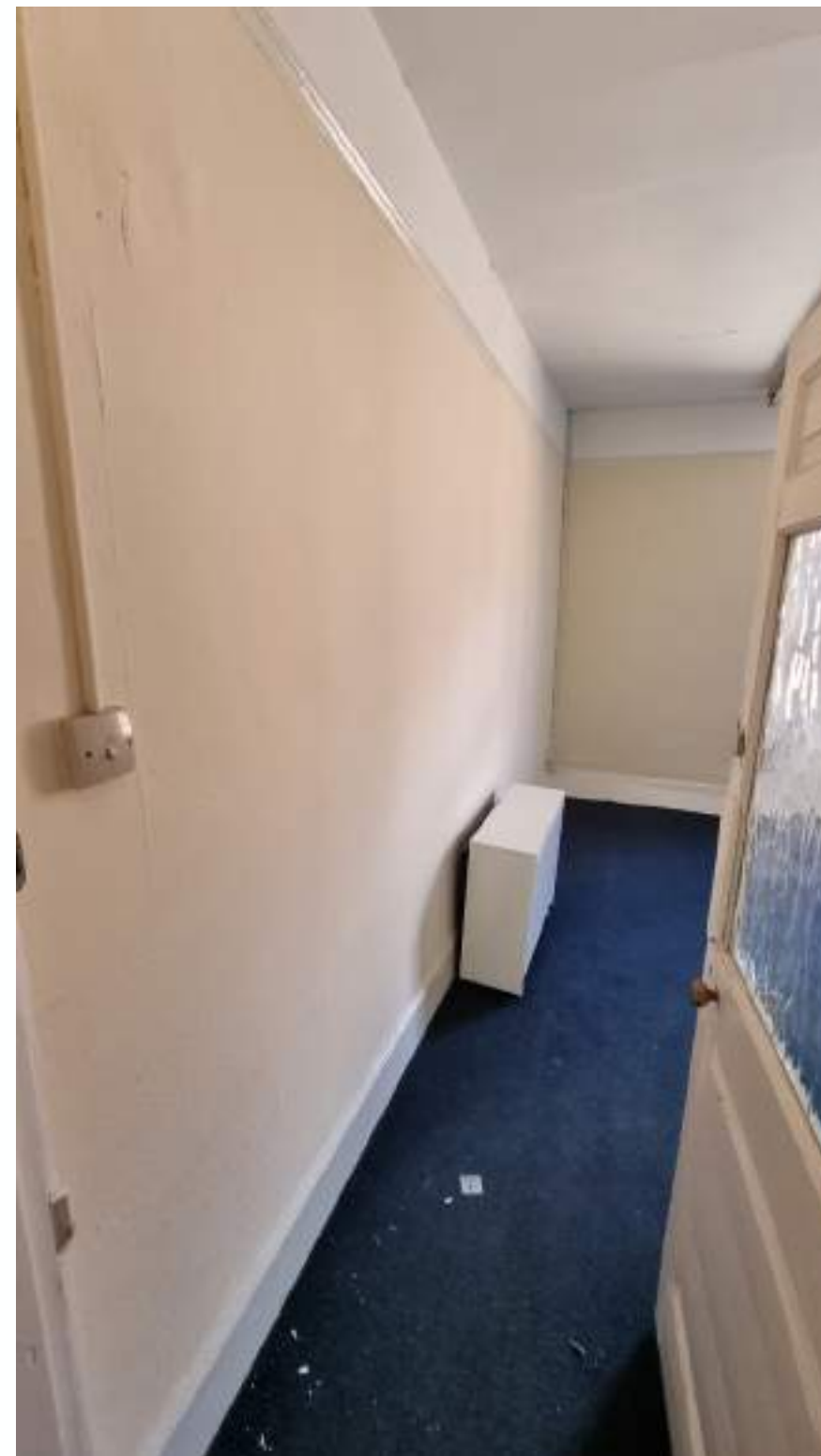
Minimal details to walls and ceiling. Modern heater to be removed
