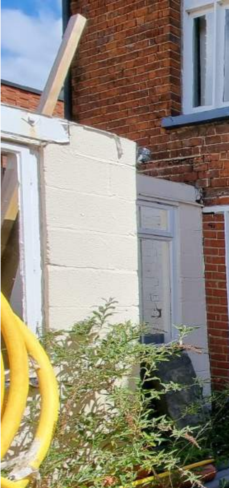
Remaining wall of mostly collapsed extension to the north - painted blockwork.
