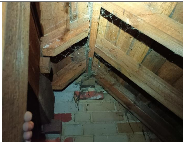
PHOTOGRAPH 14– COBWEBBING AT THE RIDGE AND GABLES
