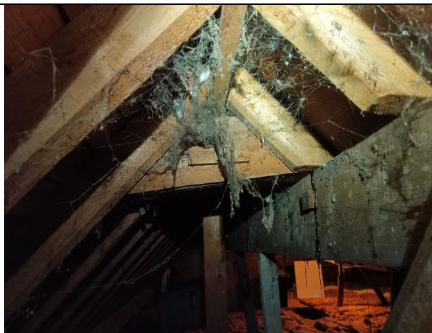
PHOTOGRAPH 13– HEAVY COBWEBBING AT THE RIDGE
