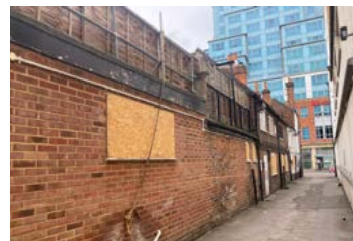
Figure 4.11 Views to and from Fife Court, showing the flank elevation of the Bugle much altered and in poor condition
