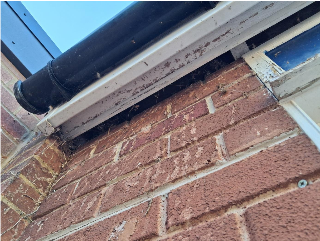
Figure 4: Gaps beneath the single-storey fascia might lead into further PRFs
