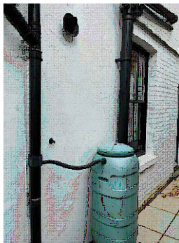
External Boiler Flue
