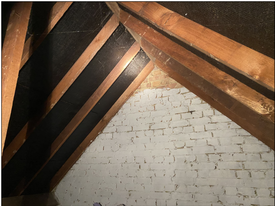
Photograph 4: Showing the cobwebbed roof space.
