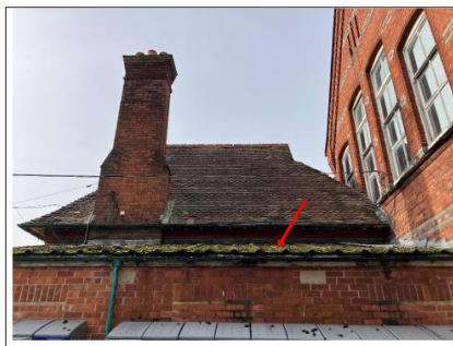
Photograph 11 Asbestos cement armory roof to be replaced
