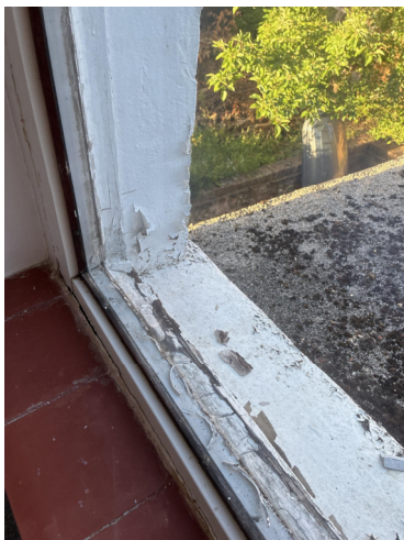
Figure 1 Window NE-1 Showing Rotten Frame
