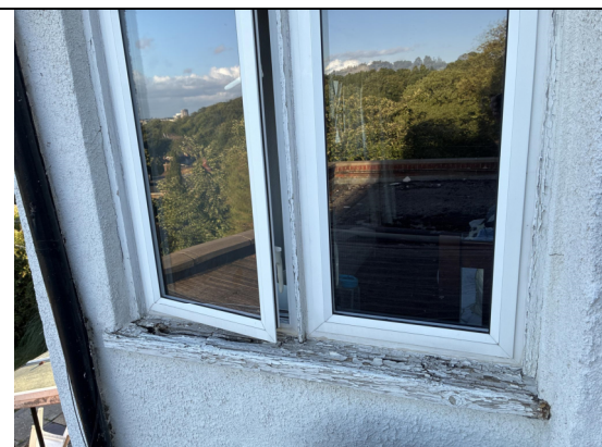
Figure 5 Extensive Damaged to Cill
