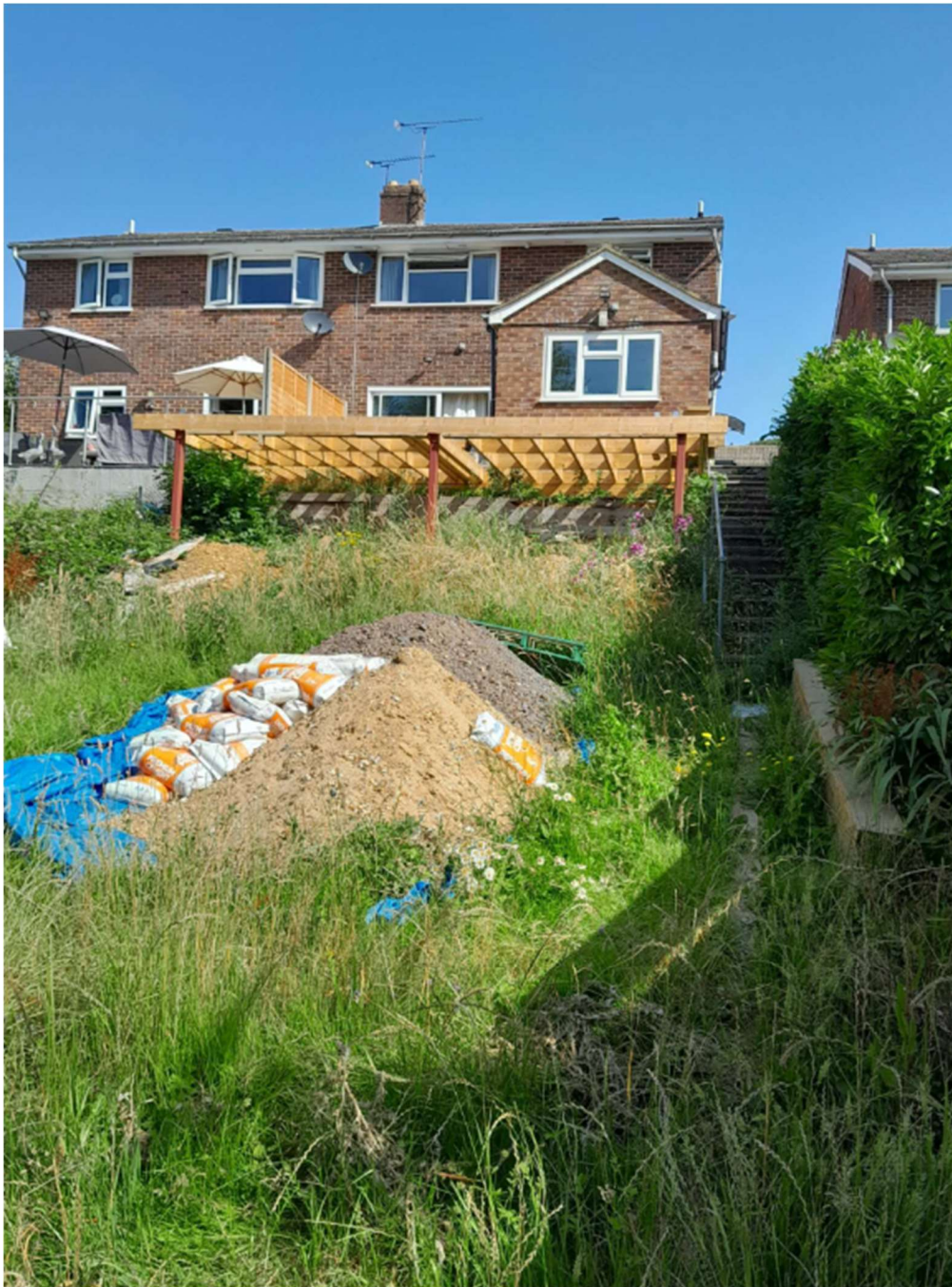
Looking north towards host property rear elevation and unauthorised decking
