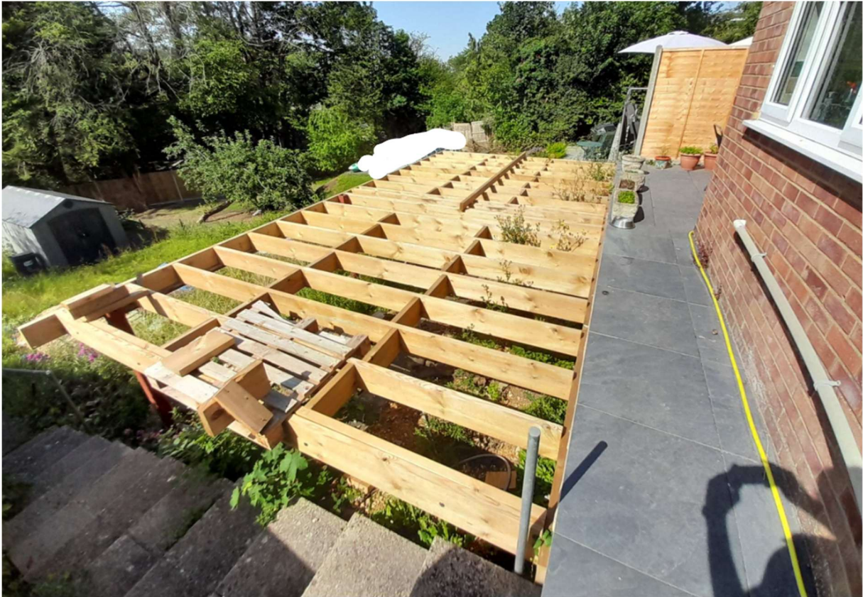
Looking west across unauthorised decking and onwards to attached neighbouring rear garden
