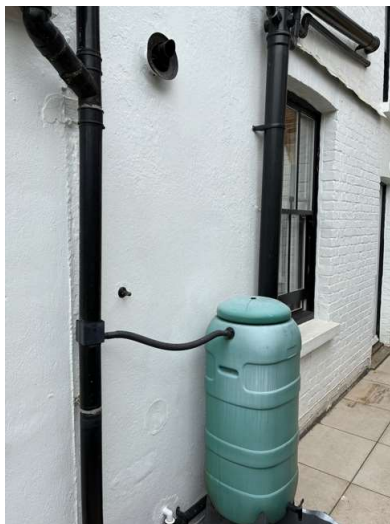
Boiler Flue location externally
