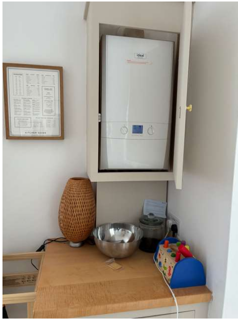
Wall Mounted Boiler 2026
