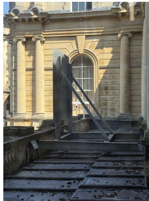
Galvanised steel support frame.
