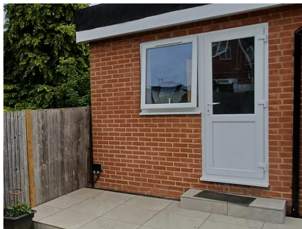
Figure 8 - Site photo showing external power point below designated flood design level
