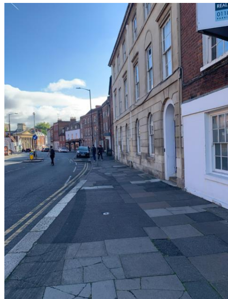
Photograph 10: Castle Street Southern Footway Conditions
