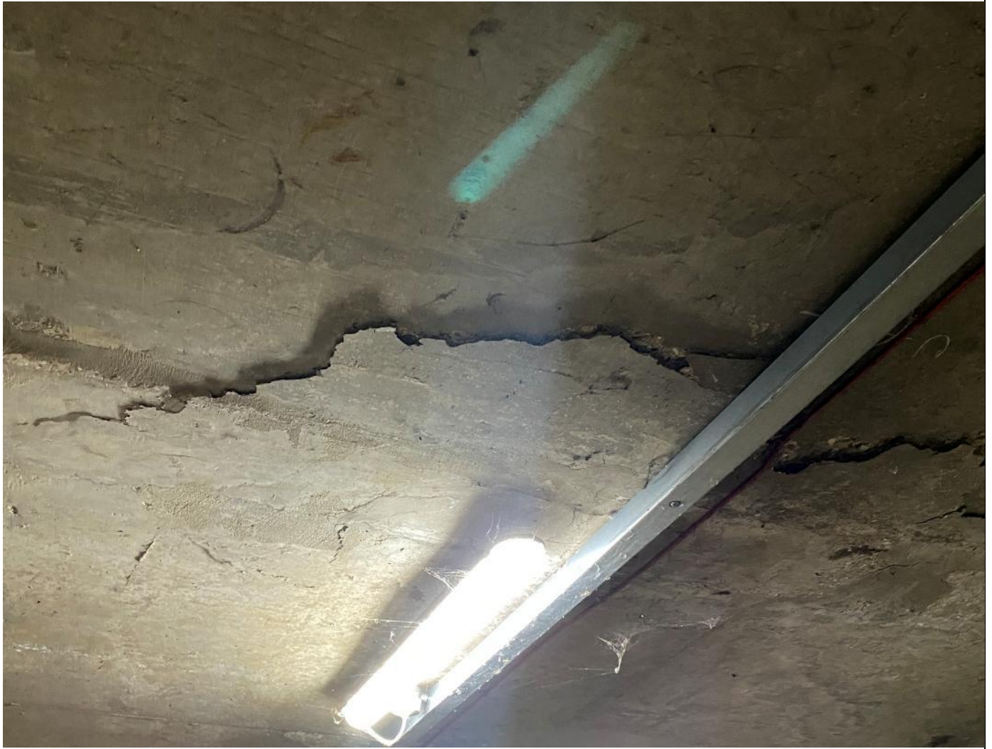
Image 2: Ceiling of basement showing visible signs of cracking
