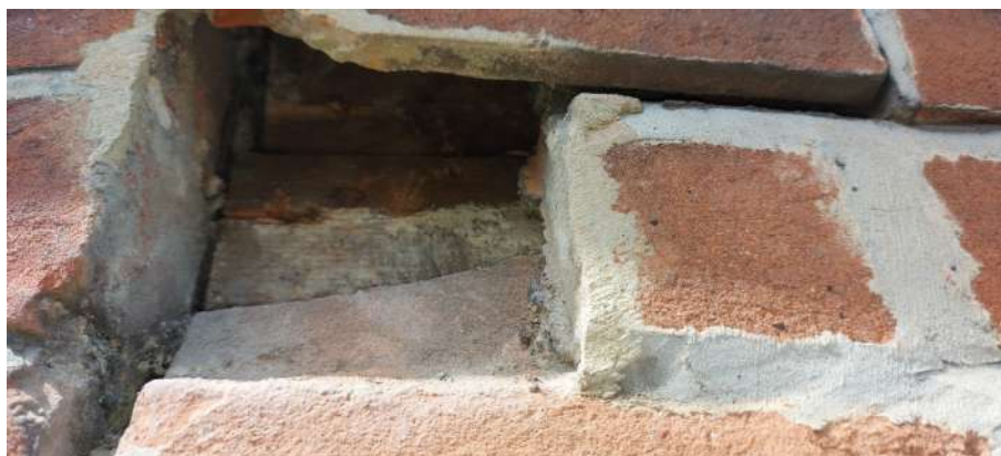
Figure 6. At south end junction with later solid wall. Timber poor
