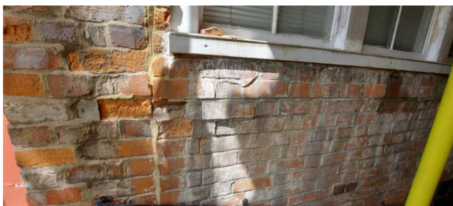
Figure 10. Ground floor – significant distortion
