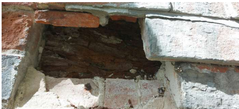
Figure 7. Ground floor – timber board very poor
