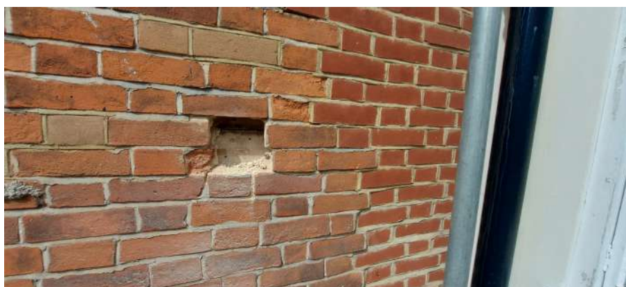
Figure 3. Top of wall – note previous rebuild on right
