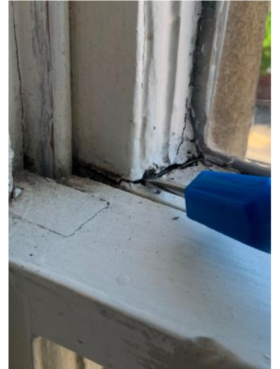
Rot to the Top sash mid rail and stile joints
