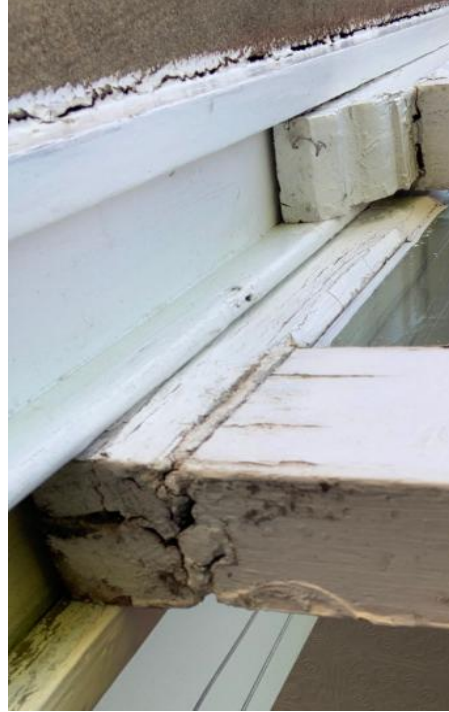
Rot to the lower sash RHS bottom rail and stile joint
