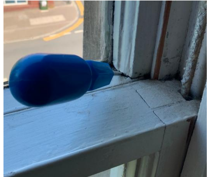
Rot to the Top sash RHS mid rail and stile joint
