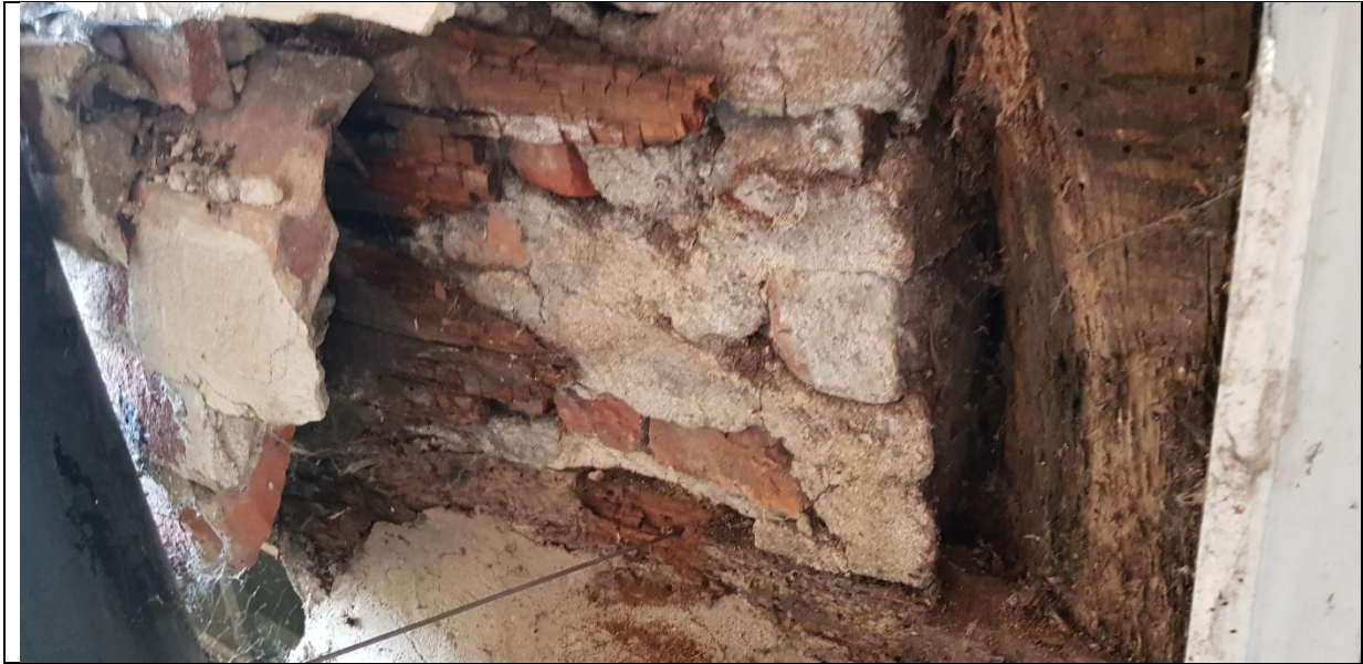
Photograph 7 Decayed cill with probe in place and decayed stud/door framing to right. Note cementitious render to face of cill
