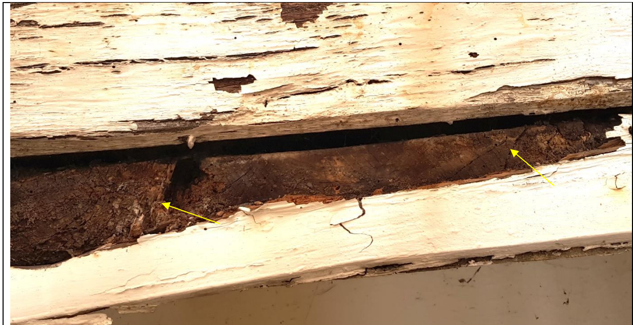
Photograph 2 Timbers beneath lintel showing fractures associated with slope of grain (arrowed) with extensive decay/failure of overlying timber fixed to its face
