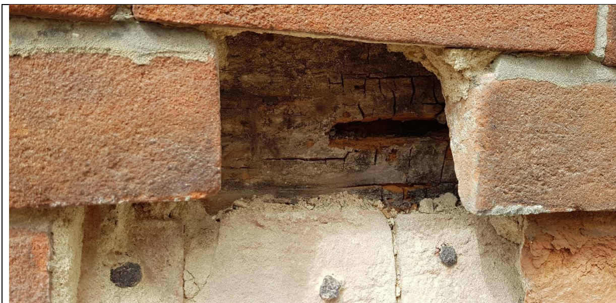
Photograph 4 Board showing extensive but historic brown rot attack (cuboidal cracking and red brown colouration of wood)
