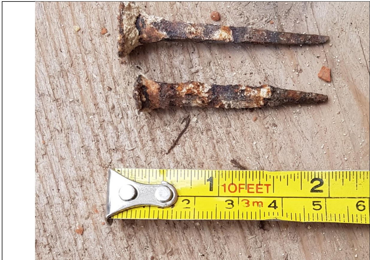
Photograph 6 Corroded fixings for engineered tiles indicating boards through which they were fixed were of high moisture content
