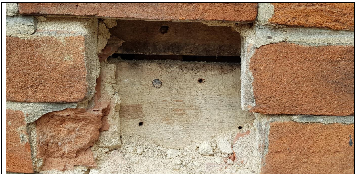
Photograph 3 Boards to which engineered tiles are fixed in good condition in this location. <20% moisture content and free from decay. Fixings show location of batten to rear.
