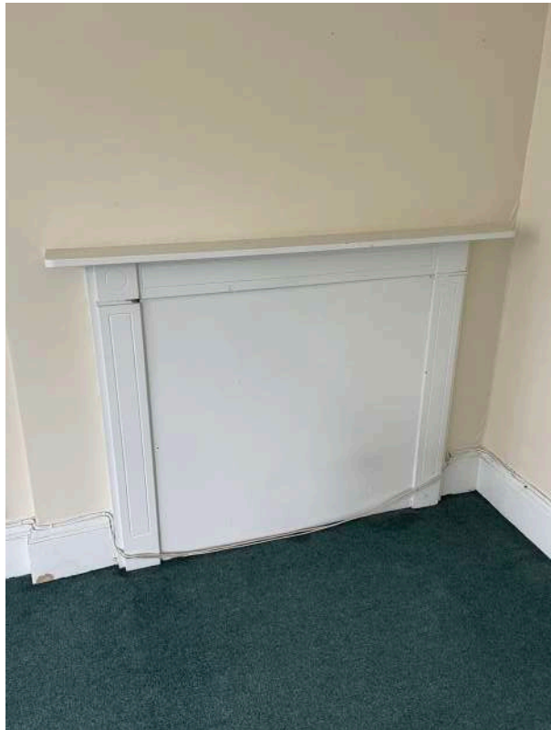
D7 - Closed-off fire surround in waiting room (13)
