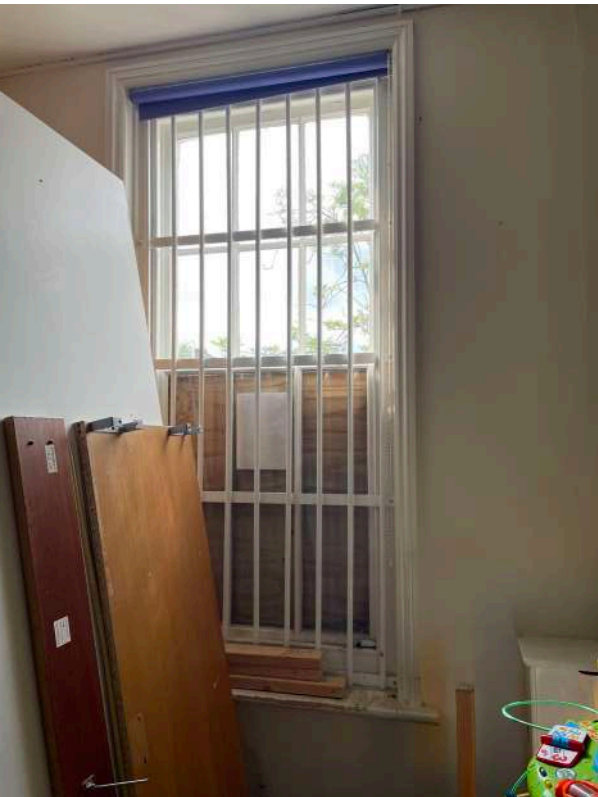
H5 - Damage timber sash window with security bars in waiting room (6)
