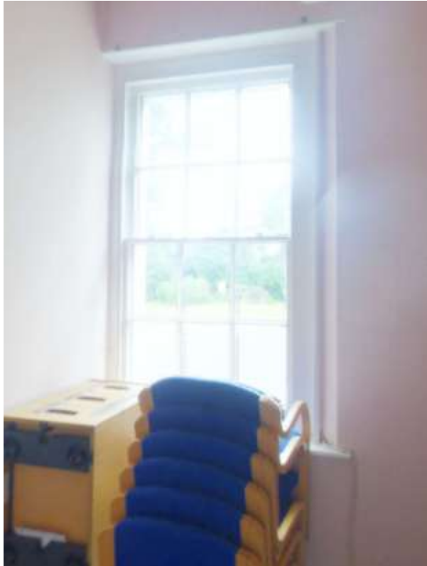
L1.3 - window surround in butler pantry (39) is far less decorative
