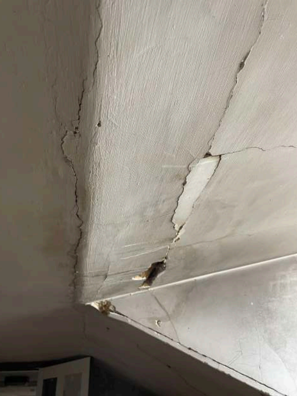
B4 - Water damage to dormer ceiling join in Eastern Storeroom (18)
