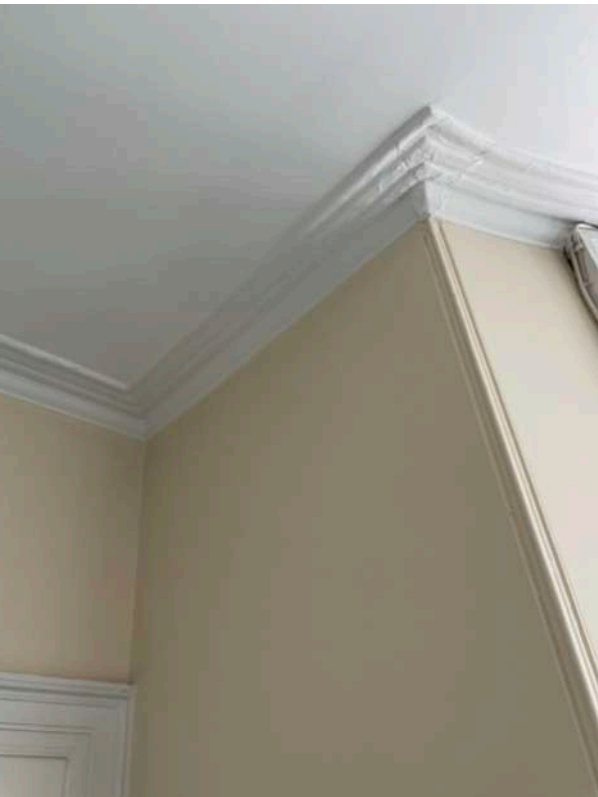
H1 - Cornice in administration office (5)
