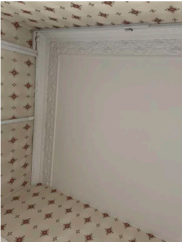
J6 - Cornice is interrupted between Corridor (2) and Deputy Office (3)
