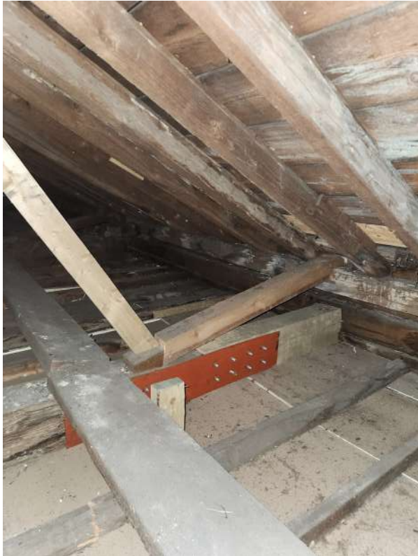
B3 - Under eaves structural timber, showing evidence of repaired (17)
