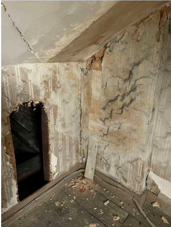
B2 - Water ingress through ceiling and damp penetration and opening to walls in western SR (17)
