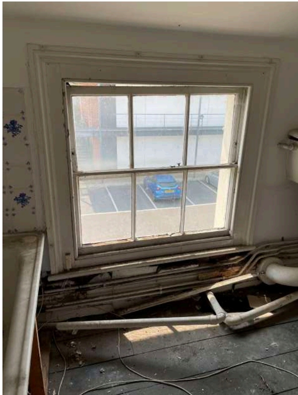
03.2 - Services running below window in bathroom (33)
