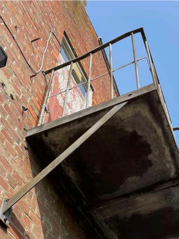
T4 - Eastern first floor fire exist to become internal access within unit 8.
