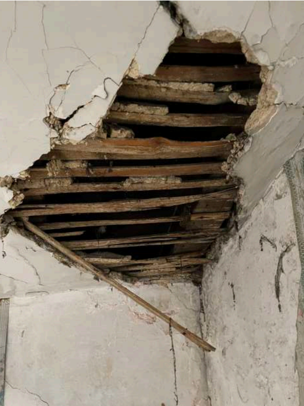
B1 - Ceiling lath and plaster destroyed by leak in eastern storeroom (18)
