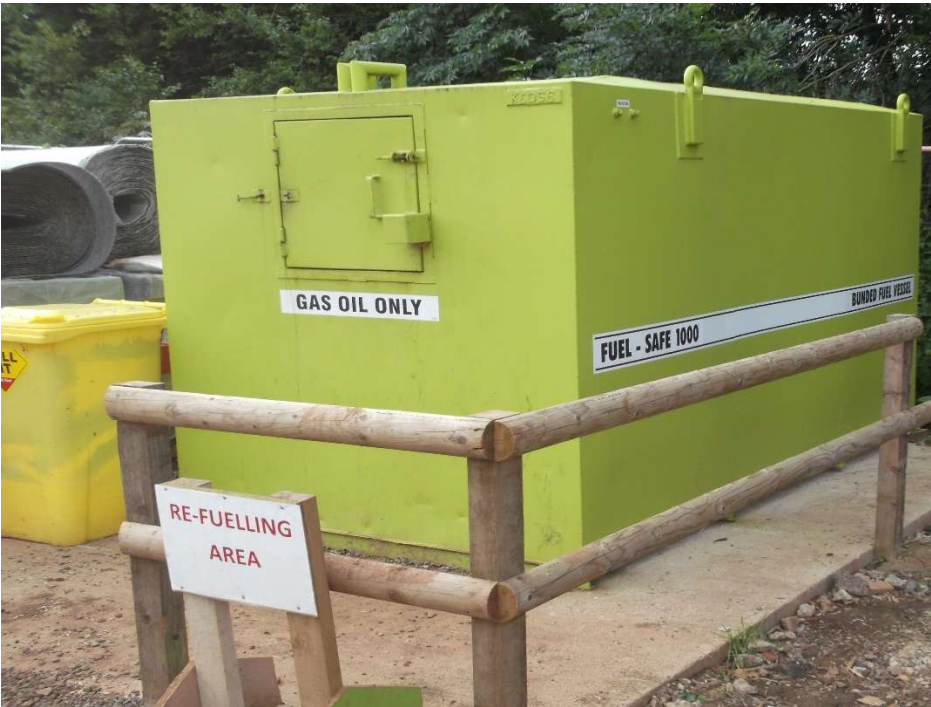
Figure 5 - Example of a protected refuelling area on handstand with spill kit
