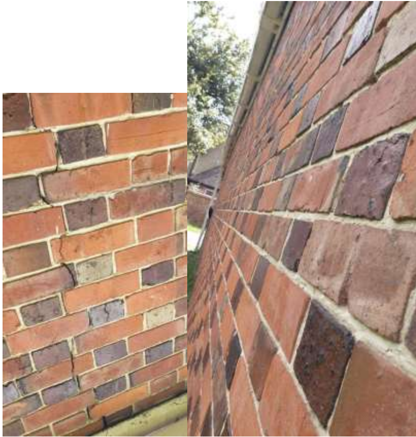
(Tilted & cracked wall of garage)
