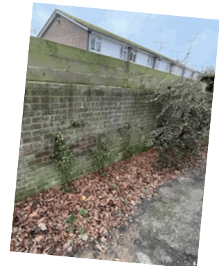
f. Damaged Wall
