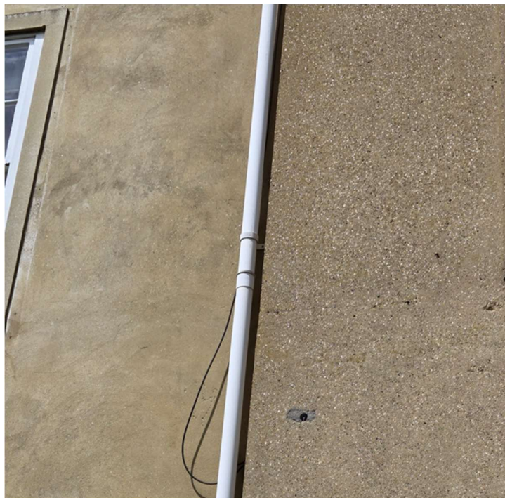
138 Castle Hill (Left) compared to 136 Castle Hill (Right) showing proposed finish vs damage/wear
