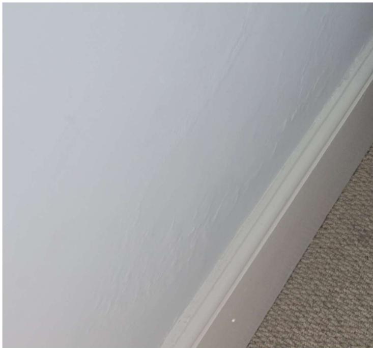
Internal photograph showing damage from water ingress
