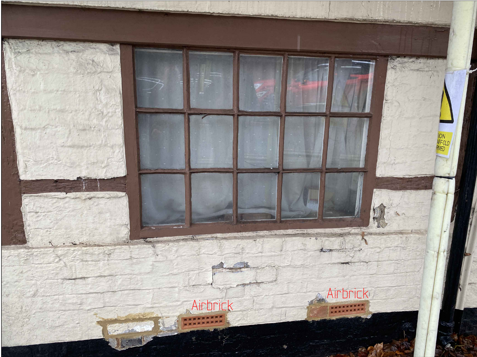
The installed airbricks in-situ - NTS
