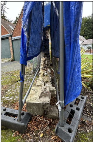
07 Stable Gateway - Damaged Wall NTS
