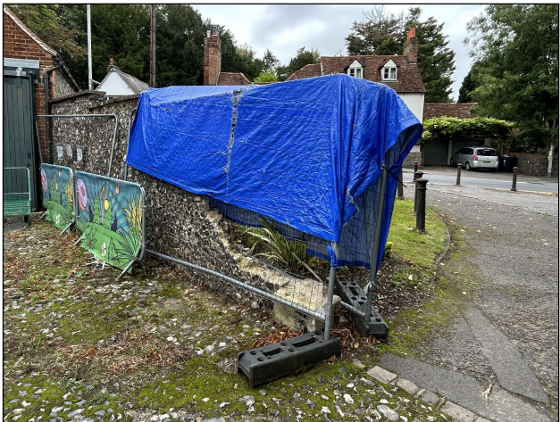
06 Stable Gateway - Damaged Wall NTS
