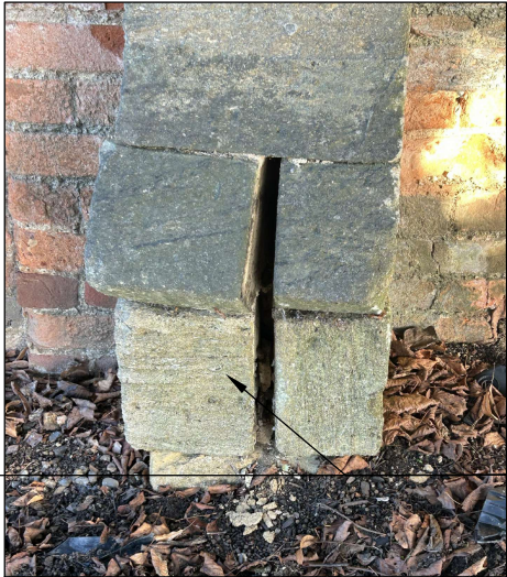
03 Boundary Wall - Damaged Pier Base NTS
