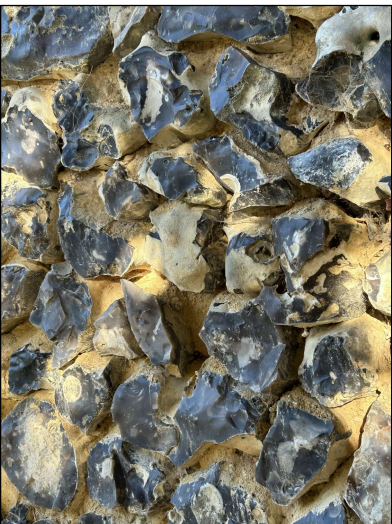
04 Boundary Wall - Loose Flints NTS
