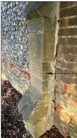
05 Boundary Wall - Damaged Pier NTS
