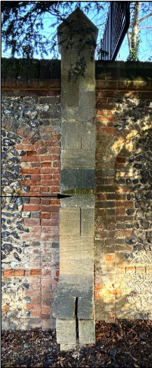
06 Boundary Wall - Damaged Pier NTS
