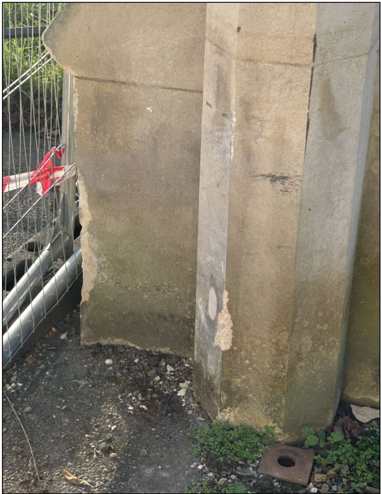
03 Damage to Gate Opening Reveal NTS
