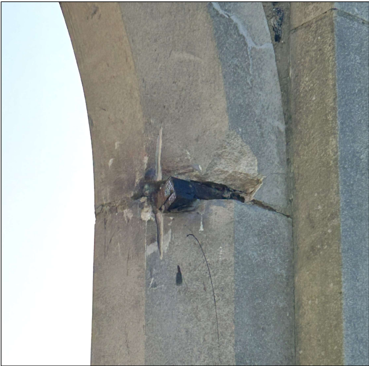
04 Damage to Hinge Pin NTS
