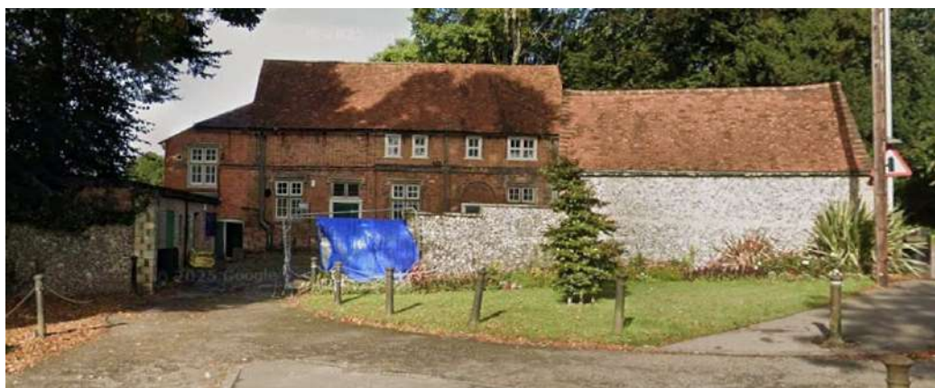
Stable Block – east boundary wall and gate piers before and after vehicle impact damage
