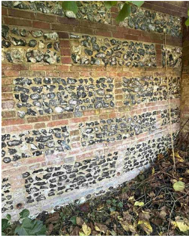
Raised Walk (Causeway) – west facing retaining wall towards the south end. View showing 'bulging brick and flintwork panel.
