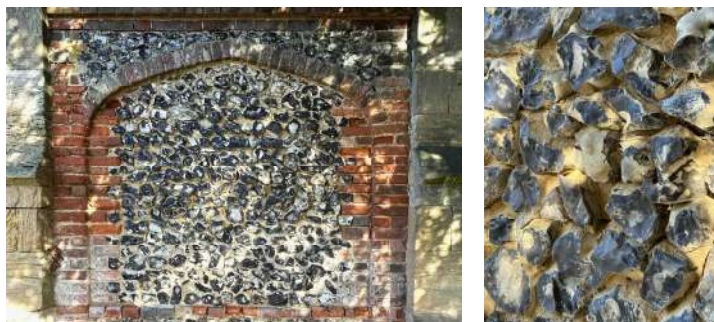
Courtyard Forecourt North Wall: defective flintwork – weathered and recessed mortar pointing and perished mortar bedding leading to loose/detached individual flints with some flints falling from the wall surface.
