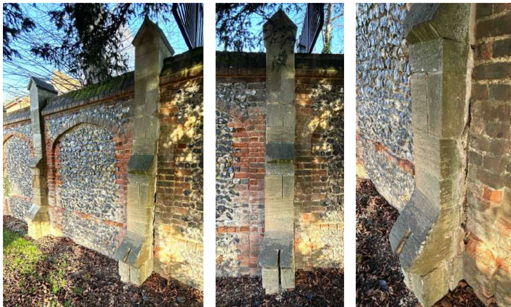
Courtyard Forecourt North Wall: damaged sustained to the natural stone ashlar block buttresses caused by vehicular impact.
