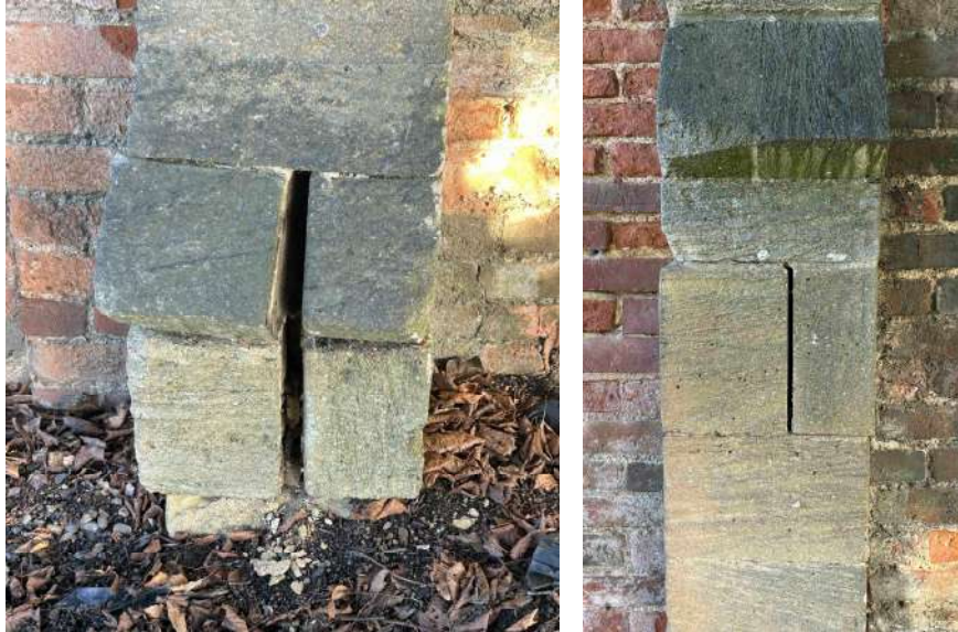
Courtyard Forecourt North Wall: damaged sustained to the natural stone ashlar block buttresses caused by vehicular impact.
