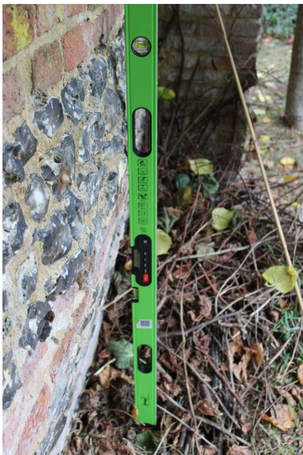
Fig. 4.5 West wall Bay 2 bulge projects approx. 150mm at peak
