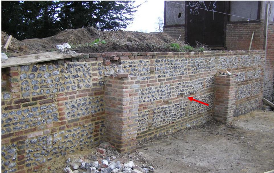
Fig. 3.11 Causeway, west wall at south end, bulge in repaired Bay 2 in 2008
