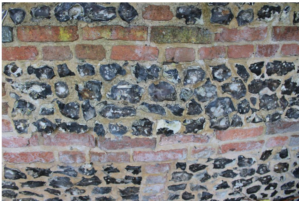
Fig. 4.6 West wall Bay 2 – local mortar cracking at peak of bulge
