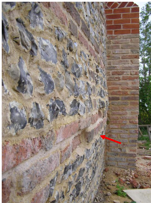
Fig. 3.12 Causeway, west wall at south end, bulge in repaired Bay 2 in 2008
