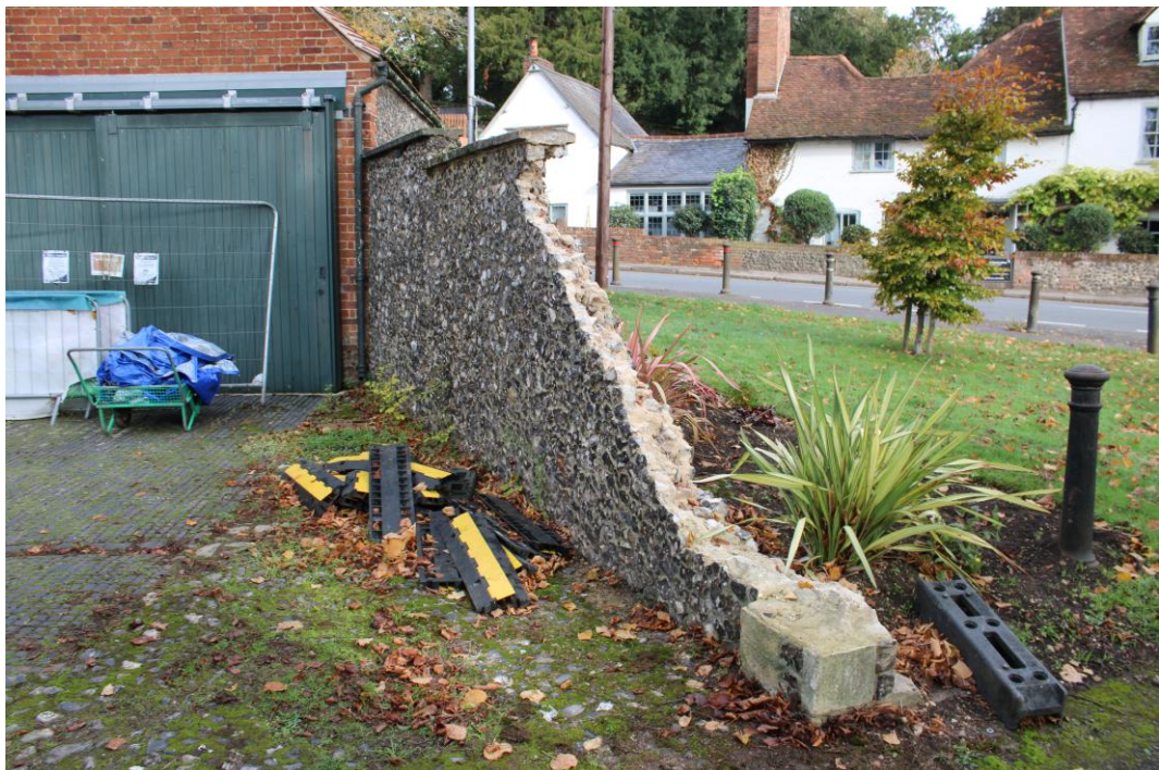
Fig. 3.1 North wall section damage from vehicle impact
