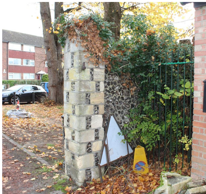
Fig. 2.4 Courtyard Wall, West elevation, part south section (undamaged)
