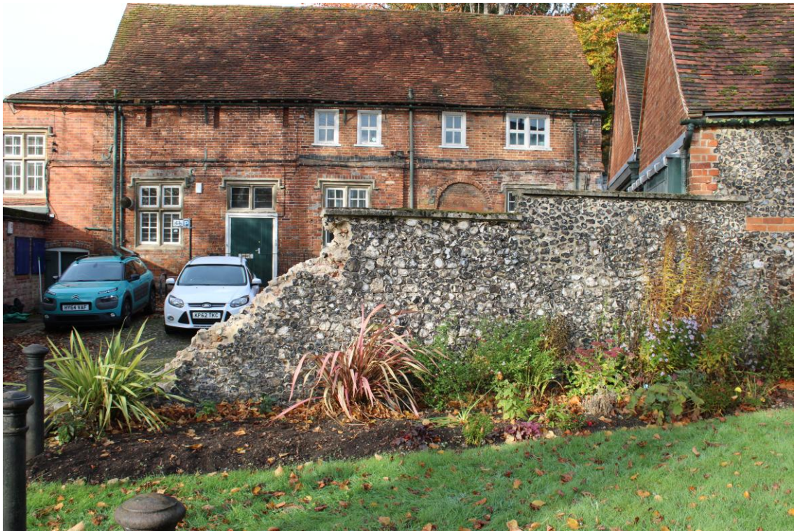
Fig. 2.2 Courtyard Wall, East elevation, north section (damaged)
