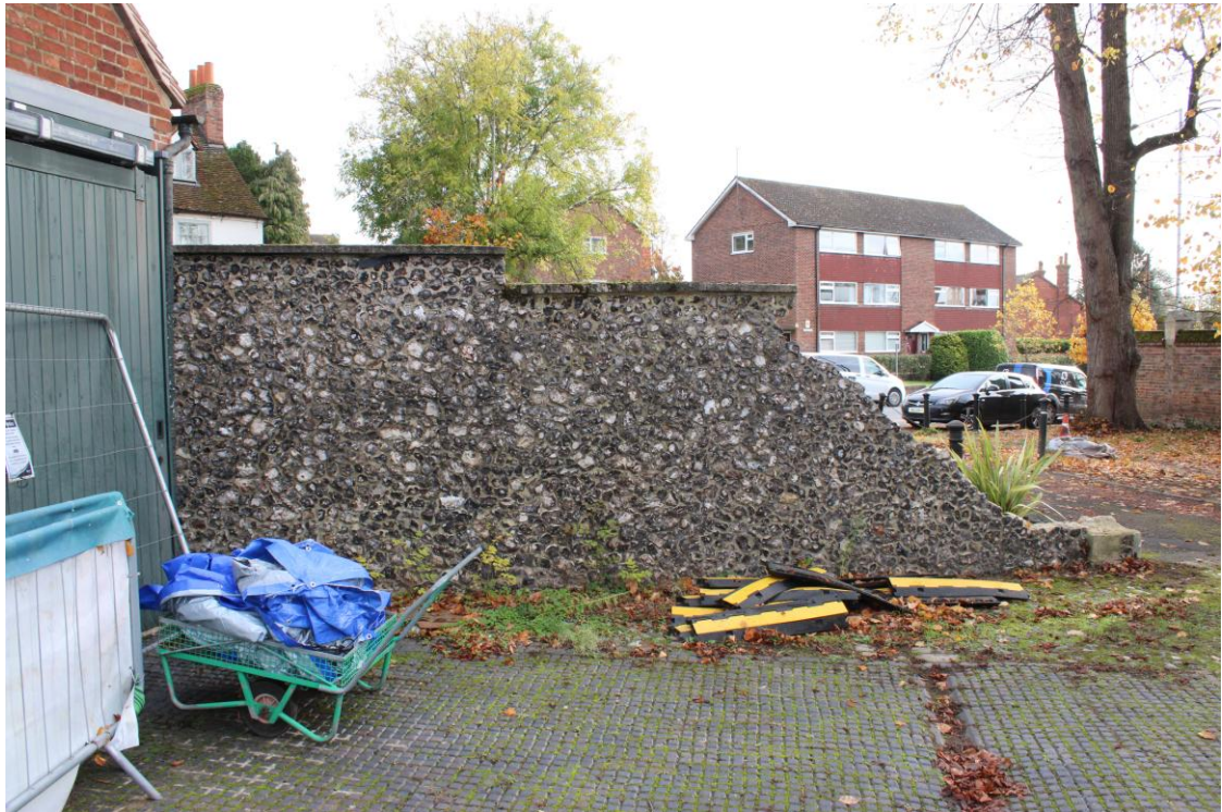
Fig. 2.4 Courtyard Wall, West elevation, north section (damaged)
