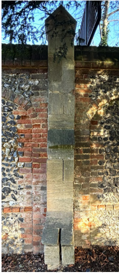
Boundary Wall- Damaged Pier
