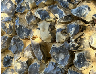
Boundary Wall- Loose Flints
