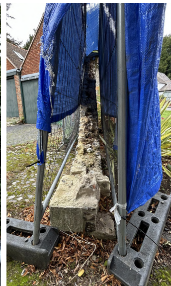
Stable Gateway- Damaged Wall
