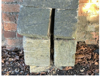
Boundary Wall- Damaged Pier Base
