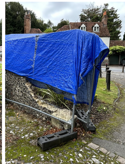
Stable Gateway- Damaged Wall
