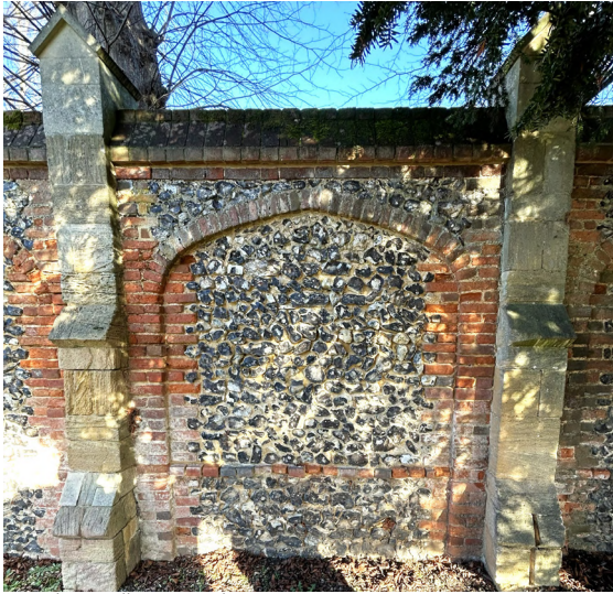
Boundary Wall- Damaged Pier
