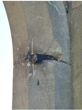
Damage to Hinge Pin
