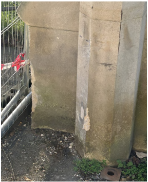
Damage to Gate Pier
