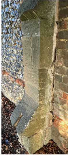
Boundary Wall- Damaged Pier
