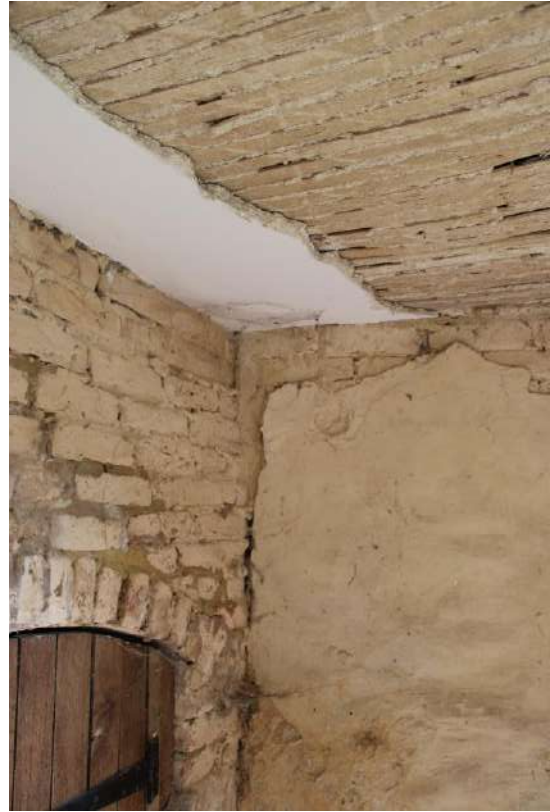
Fig. 4.30 Ground floor - northeast corner infill crack and failed ceiling
