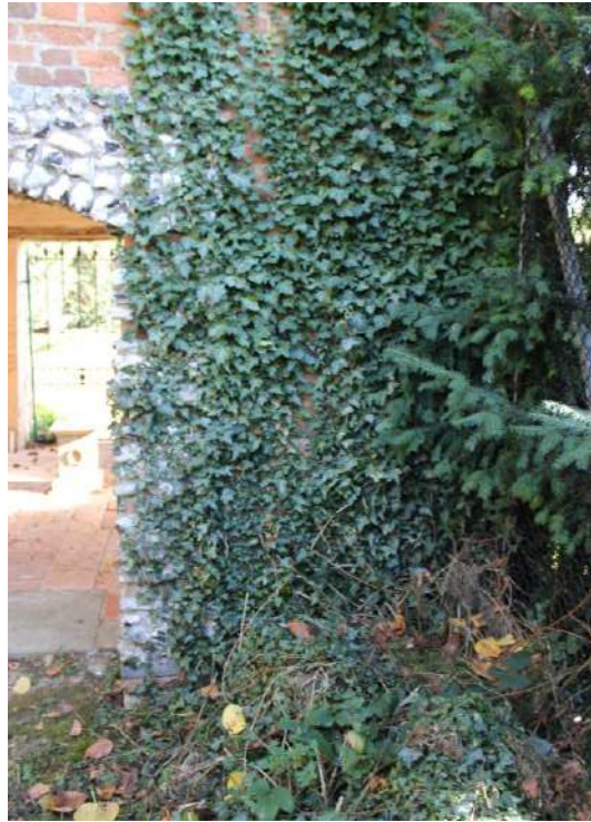
Fig. 4.22 West Elevation- ivy growth to south side
