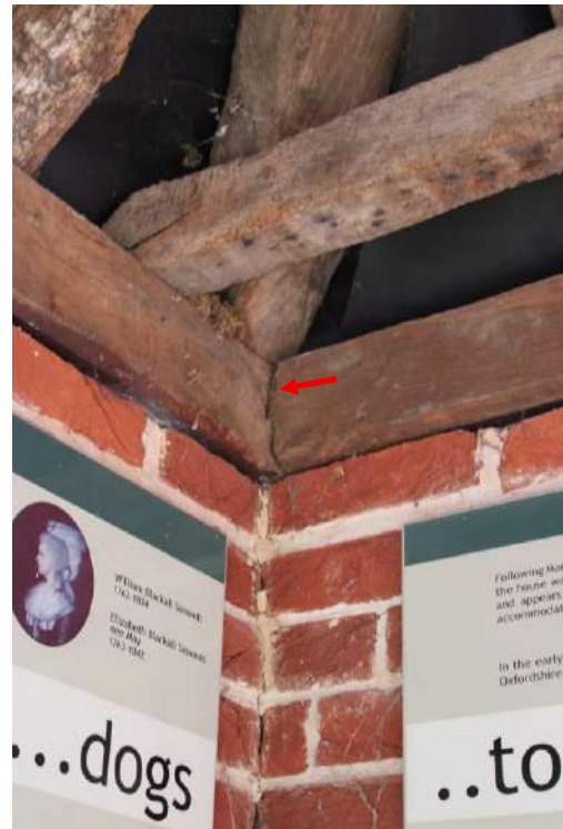
Fig. 4.43 First floor – Southwest corner upper wall plate gap
