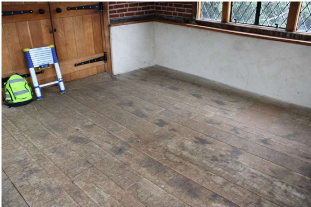
Fig. 4.49 First floor – fall in level towards northeast corner
