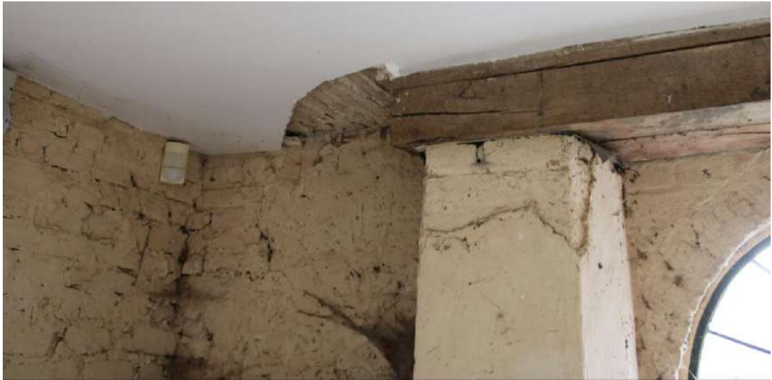
Fig. 4.35 Ground floor – south elevation – ceiling loss at east end of lintels
