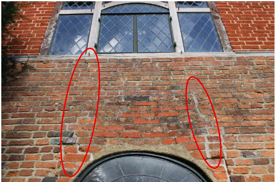
Fig. 4.18 South elevation – cracking above window
