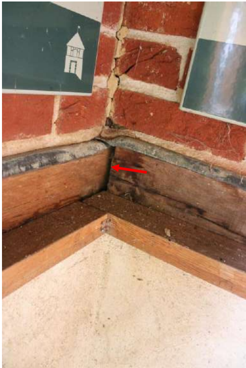
Fig. 4.42 First floor – Southwest corner lower wall plate gap
