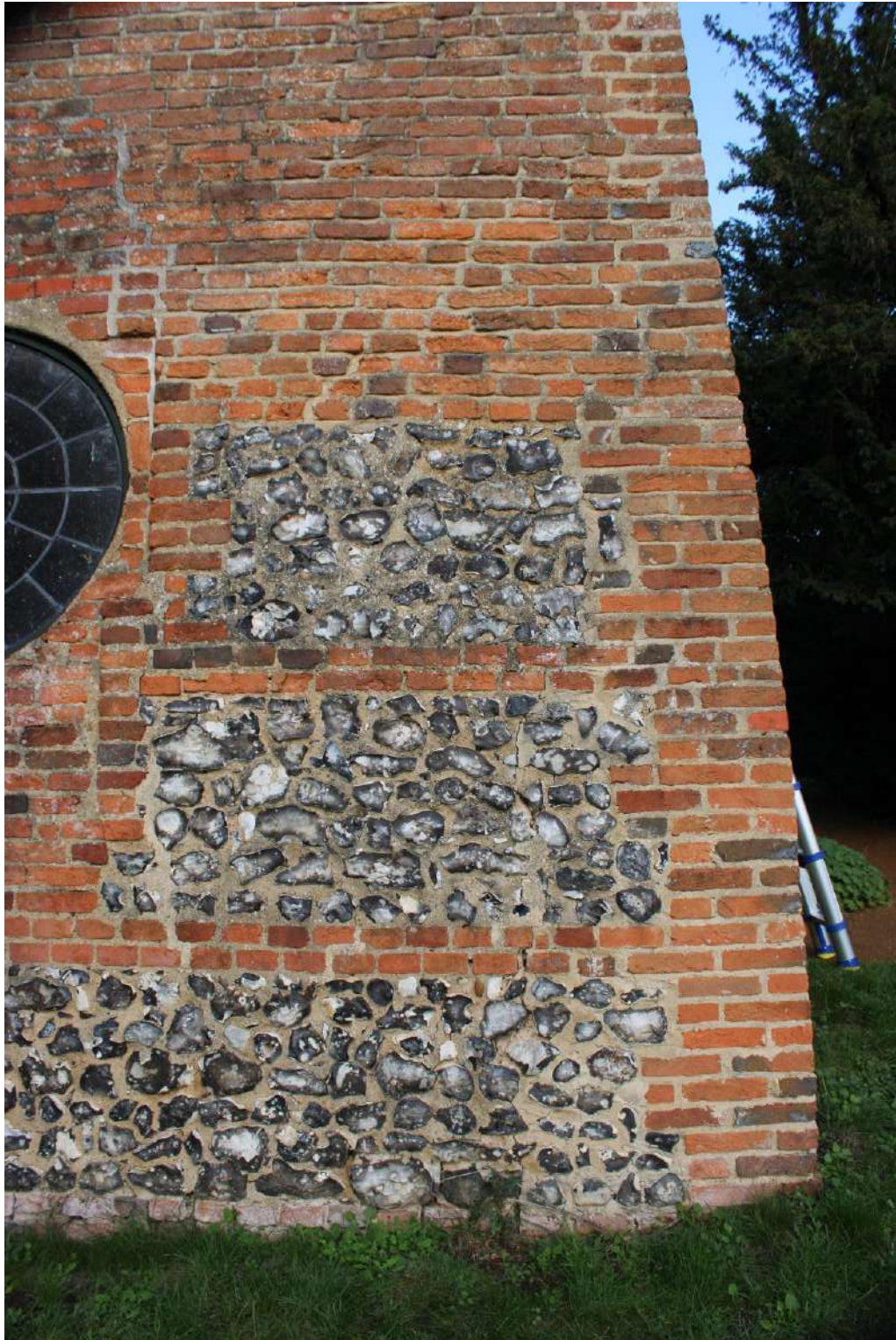
Fig. 4.14 South elevation – cracking at east corner
