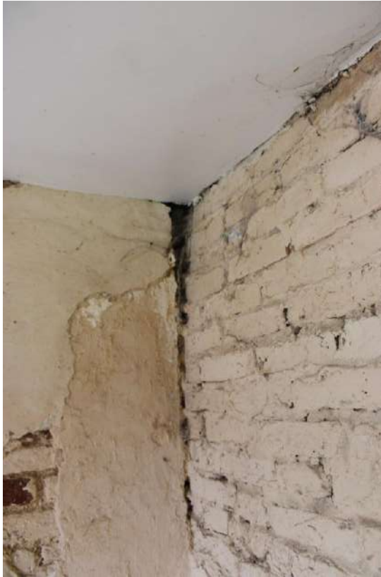
Fig. 4.29 Ground floor – northwest corner cracking
