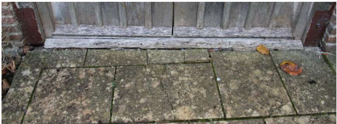
Fig. 4.1 North elevation – door sill decayed and paving defects
