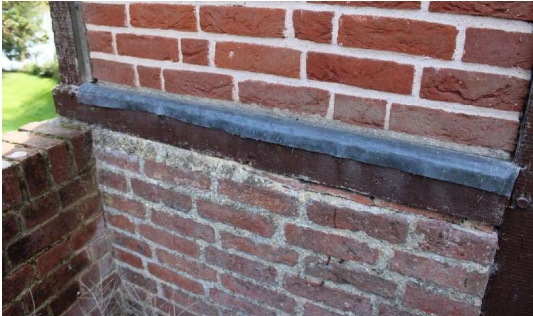
Fig. 4.2 North elevation – east wall plate with mortar loss below
