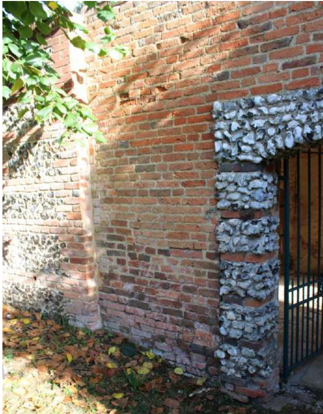
Fig. 4.24 West Elevation- mortar loss at bottom of wall and spalled bricks at higher level
