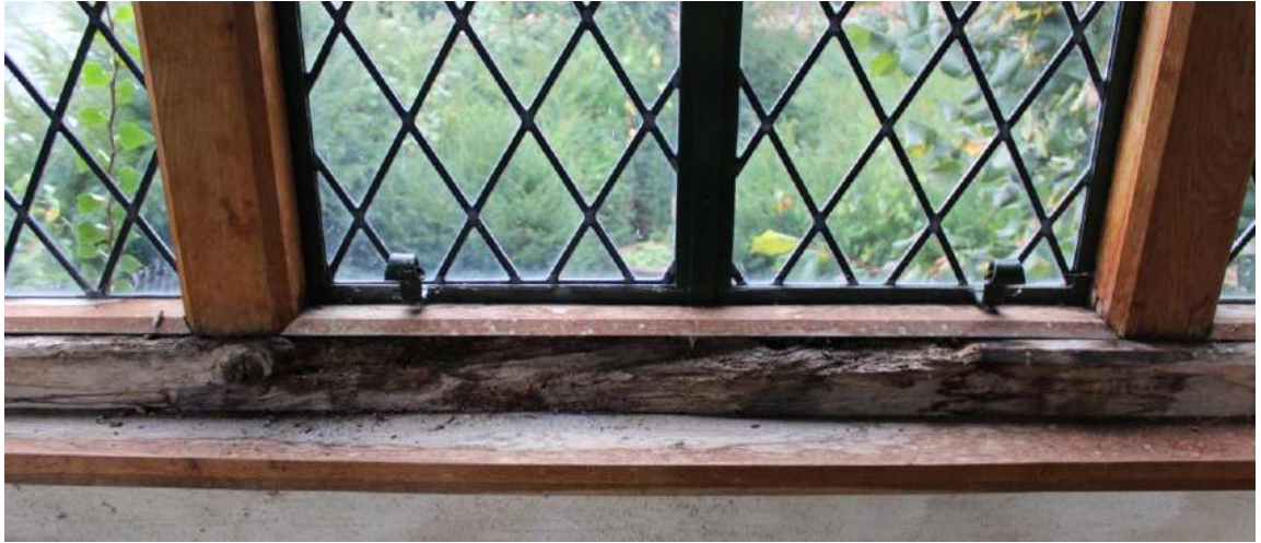
Fig. 4.48 First floor – west elevation – decay to wall plate
