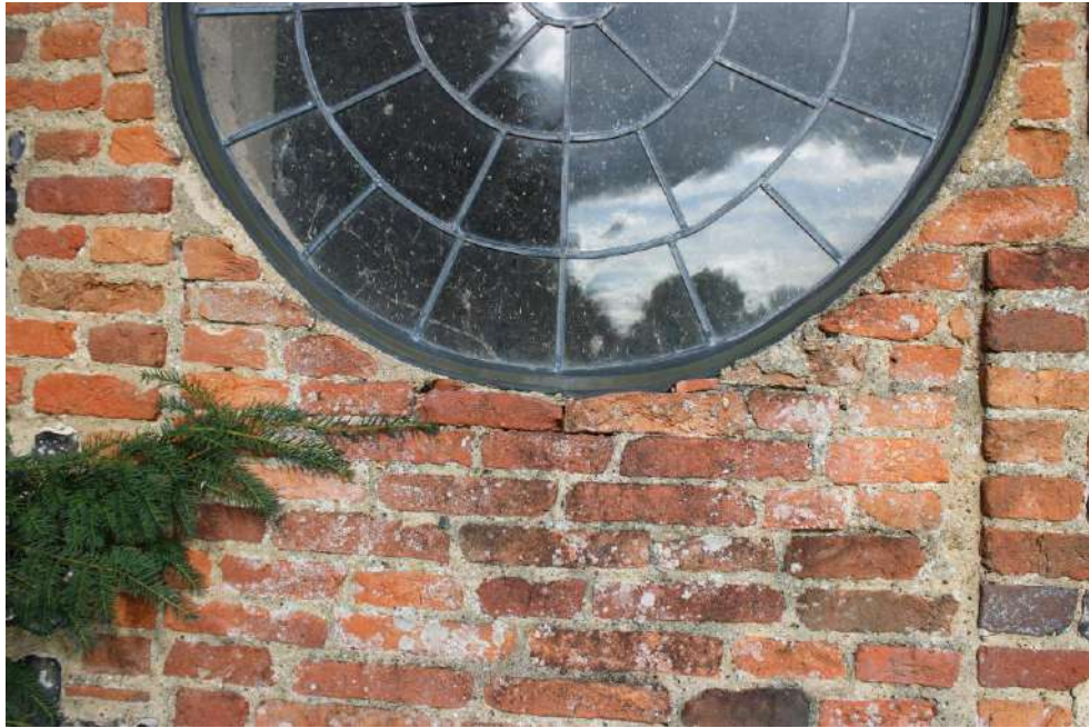
Fig. 4.17 South elevation – mortar loss below window
