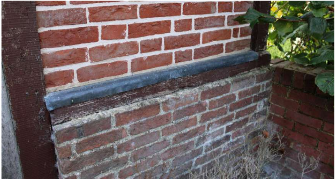
Fig. 4.4 North elevation – west wall plate with mortar loss below
