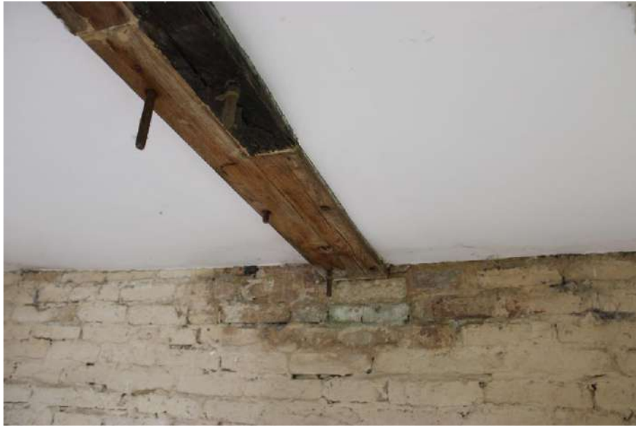
Fig. 4.31 Ground floor – previous repair to north end of main beam
