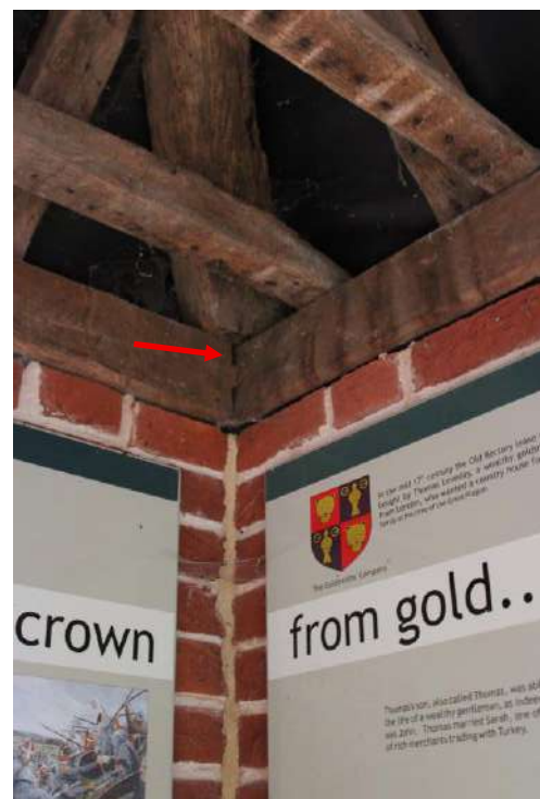
Fig. 4.45 First floor – Southeast corner upper wall plate gap
