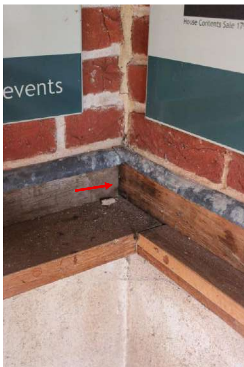
Fig. 4.44 First floor – Southeast corner lower wall plate gap
