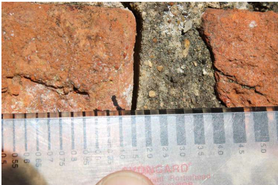
Fig. 4.16 South elevation – vertical crack, 1.5mm wide at 1580 mm high above ground.
