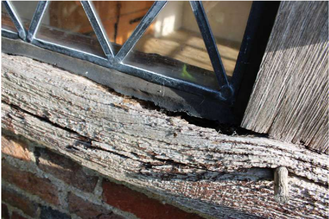
Fig. 4.26 West elevation – decay and bowing of wall plate
