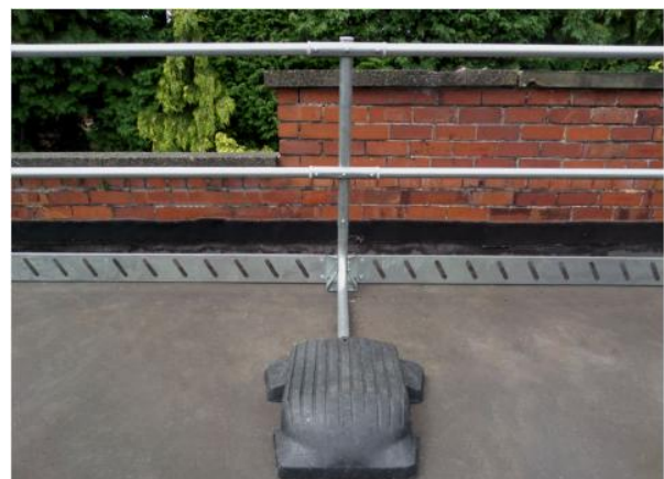
(Image of safety handrail)
