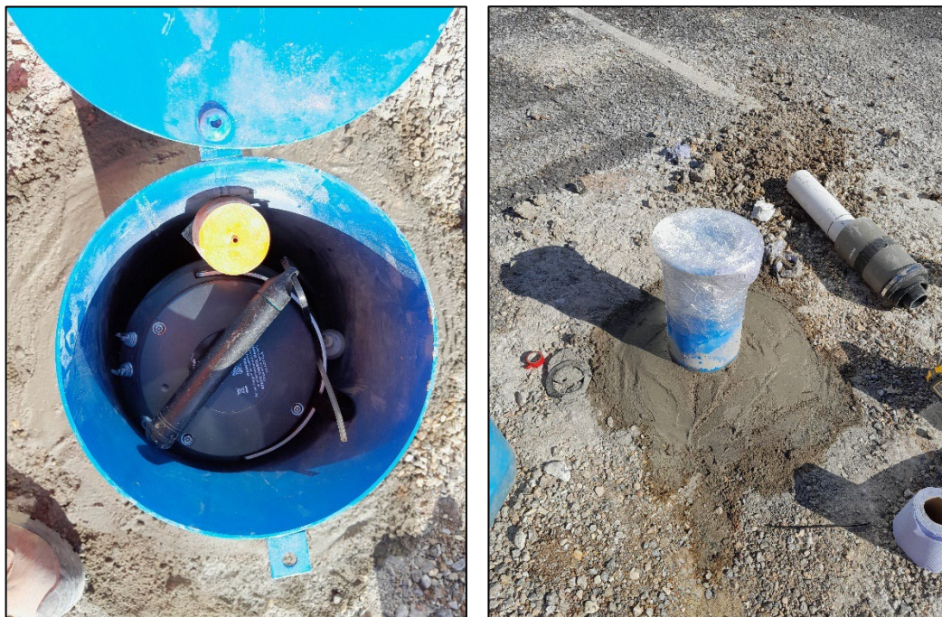
Figure 2 Selected GGS site photograph of a Gas Sentinel® continuous ground gas monitoring instrument deployed and secured on site.
