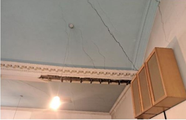
Photo 3 evidence of cracking from the 2085 Design and Heritage statement, Fusion Heritage
