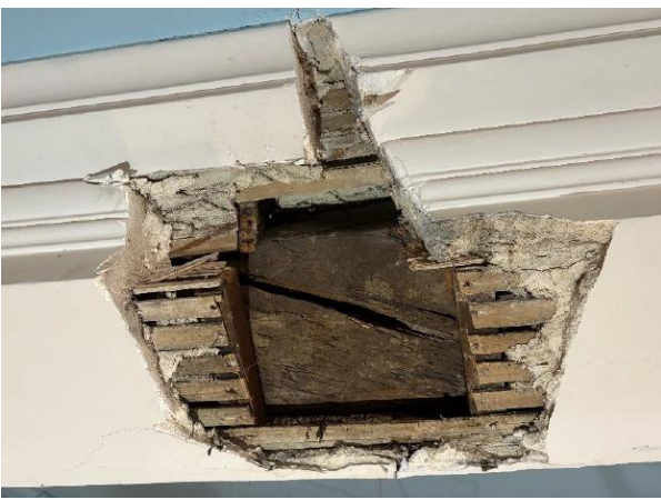
Internal photo of the beam from the structural report Fig 11, p8, Clive Hudson Associates
