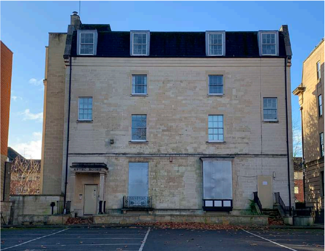
2 The rear elevation is more severe than the front elevation. There are visible alterations to the high level stonework and alterations to create the lift shaft are apparent to the lefthand set back portion.
