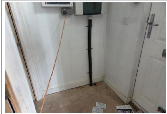
Electrical service entry
