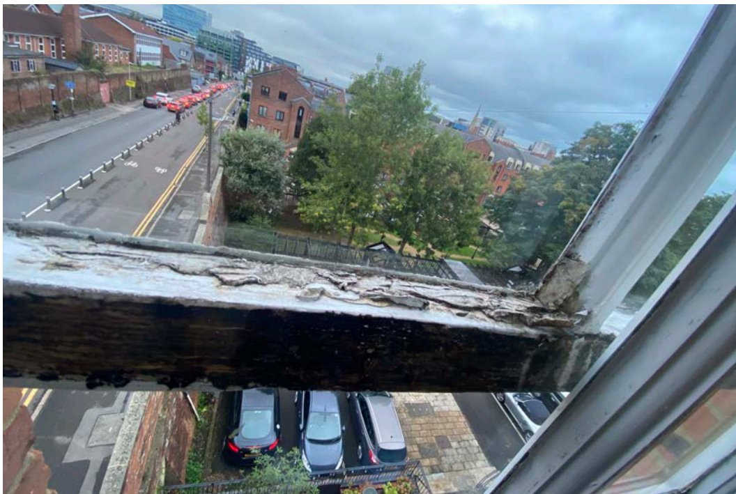
Fig.7: Rot to upper sash glazing bar junction with lower rail
