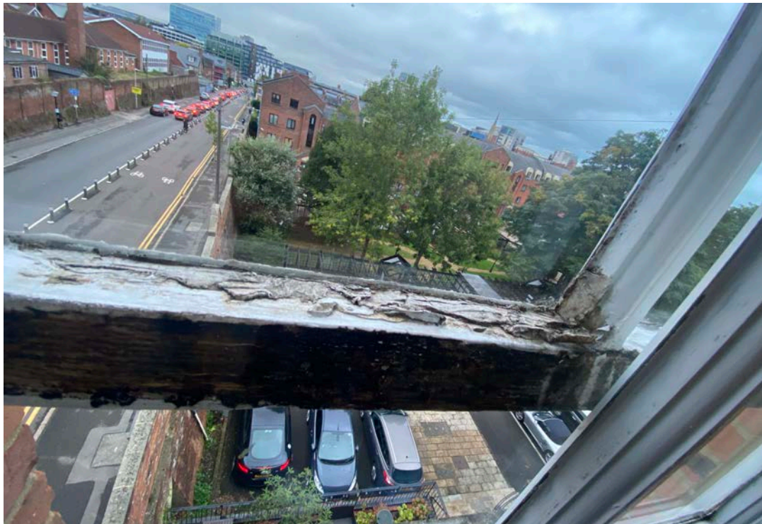
Fig.2: Rot to top sash lower rail
