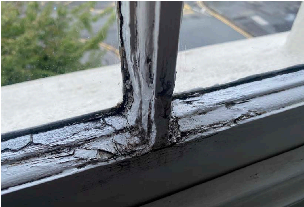
Fig.6: Rot to lower sash glazing bar junction
