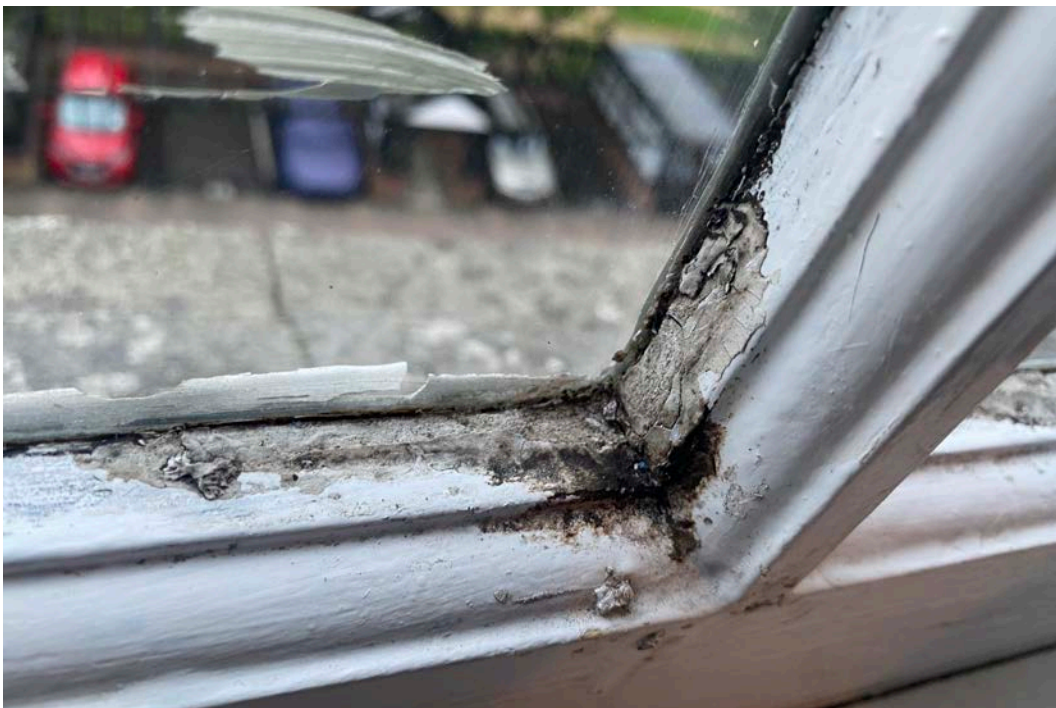
Fig.5: Rot to lower sash lower rail at glazing bar junction
