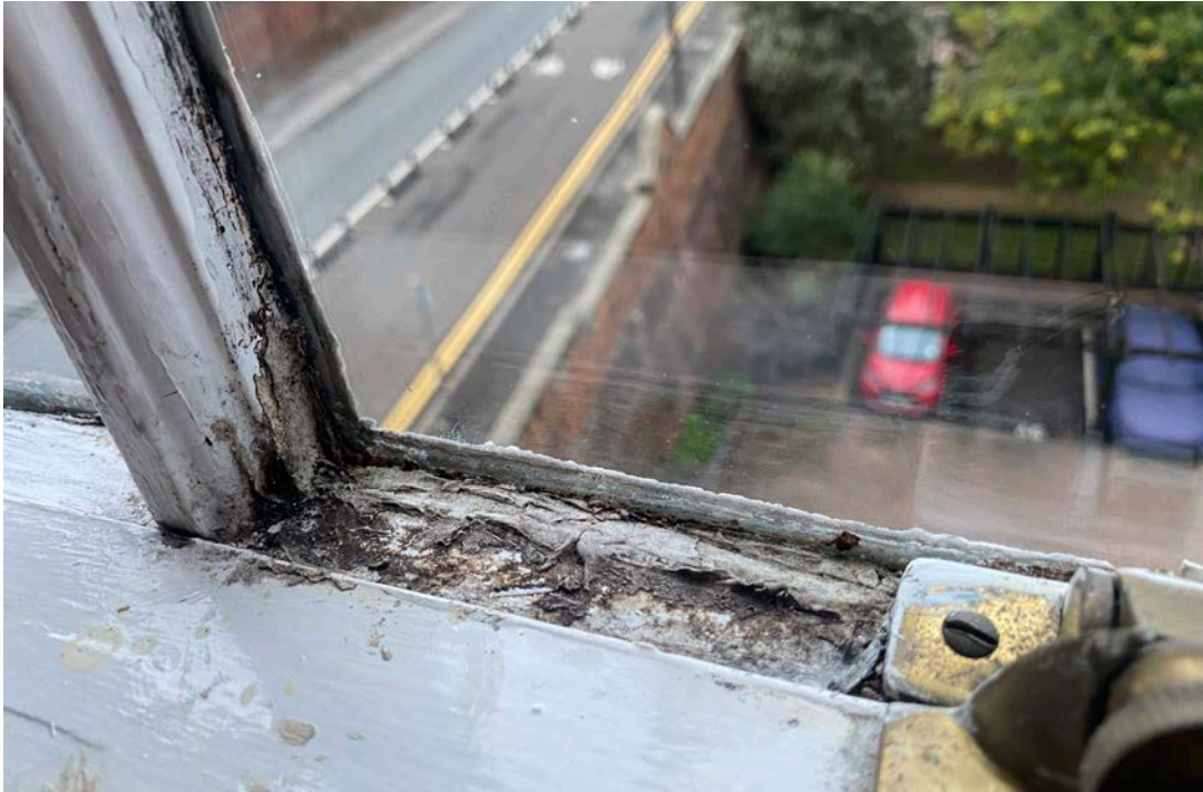
Fig.4: Rot to top sash lower rail
