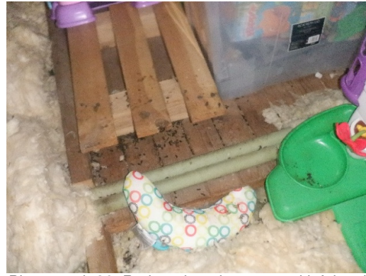
Photograph 26. Rodent droppings around loft hatch (roof void).
