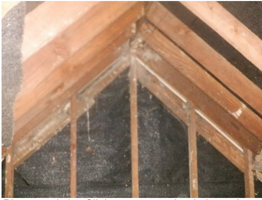
Photograph 25. Slight gaps over the timber rafters at the front gable end (roof void).
