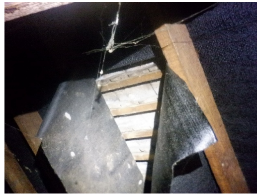
Photograph 20. Section of loose fitting bitumen felting where external roof tiles visible (roof void).
