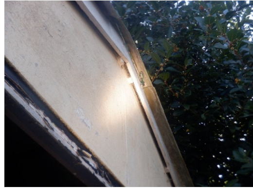
Photograph 18. Gap between the timber fascia and rendered brickwork of the outbuilding (front elevation).
