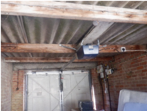
Photograph 27. Open roofed garage with large gap around the garage door (internal view of garage).
