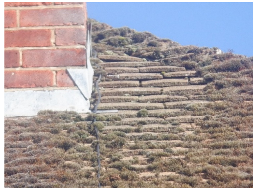
Photograph 10. Slightly lifted roof tiles; lead flashing flush to the plain roof tiles (front elevation).
