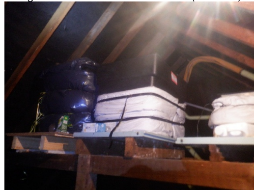
Photograph 22. Three small covered water tanks on raised platform (roof void).
