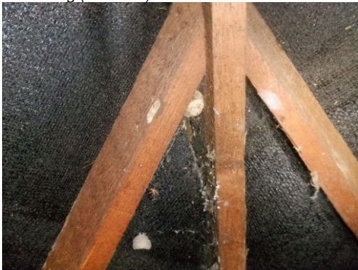
Photograph 21. Small sections of loose fitted bitumen felting (roof void).
