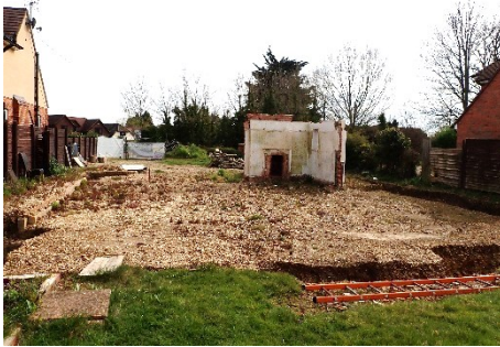
Photograph 11. Remains of house to be replaced.
