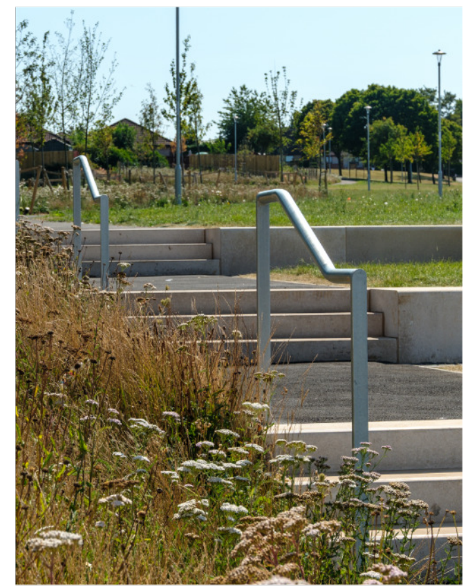
Pre-cast concrete steps & seating steps
