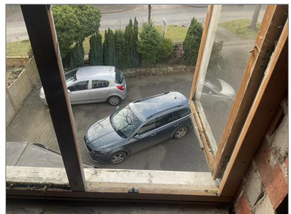
Photo - 30 Fall hazard
