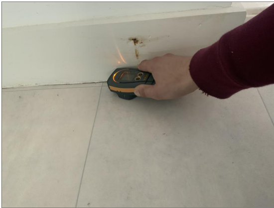
Photo - 52 Damp here
