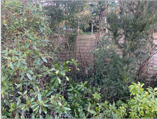
Photo - 91 Fallen over
