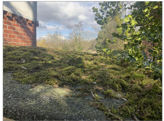
Photo - 78 Moss to roof
