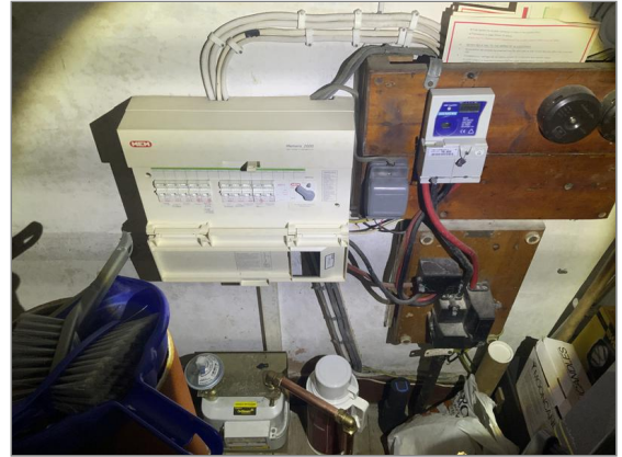
Photo - 67 Electrical fittings
