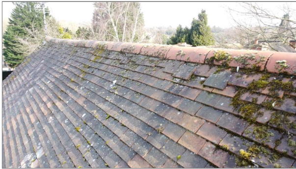
Photo - 4 Slipped tiles
