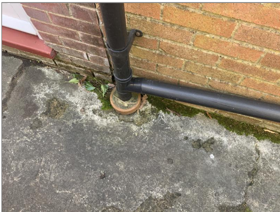
Photo - 20 Sealed system
