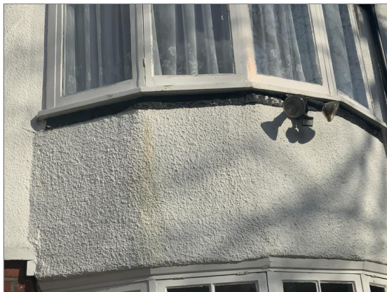
Photo - 27 Ageing flashing
