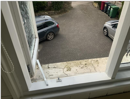
Photo - 31 Fall hazard
