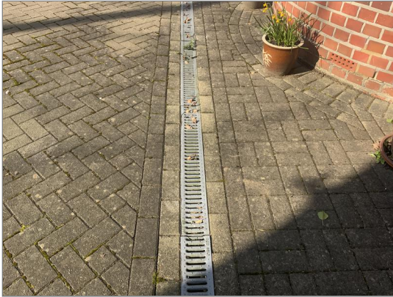
Photo - 71 Cleaning required
