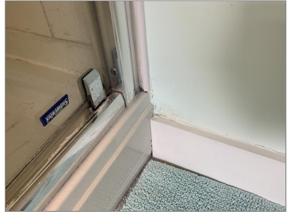
Photo - 65 Slight leak
