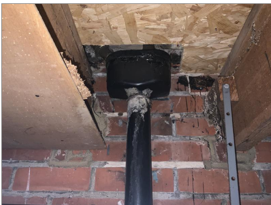
Photo - 22 Joints leak
