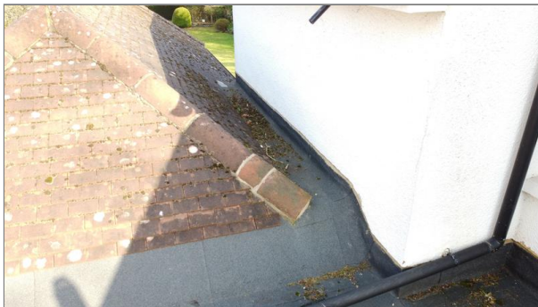
Photo - 10 Cleaning required
