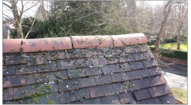
Photo - 3 Cracked ridge
