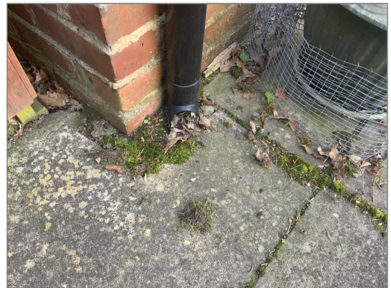
Photo - 21 Poor condition
