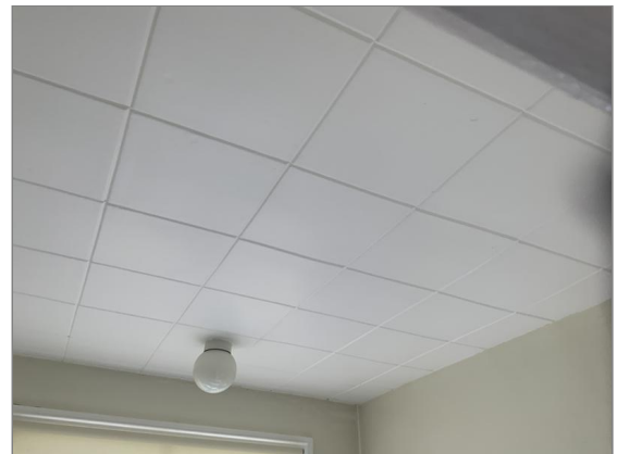
Photo - 46 Polystyrene tiles
