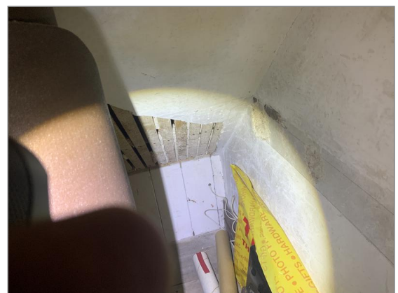
Photo - 48 Exposed laths
