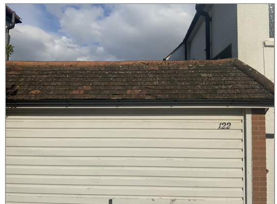
Photo - 13 Cracked tiles
