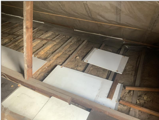
Photo - 42 Inadequate insulation
