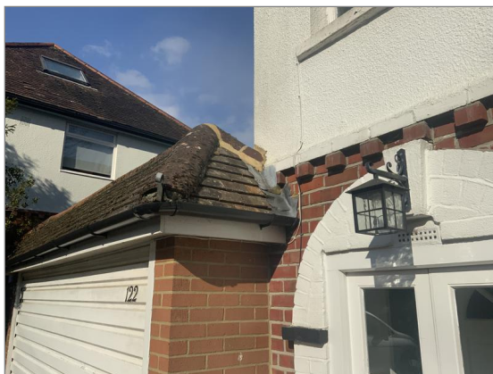
Photo - 12 Recent repair
