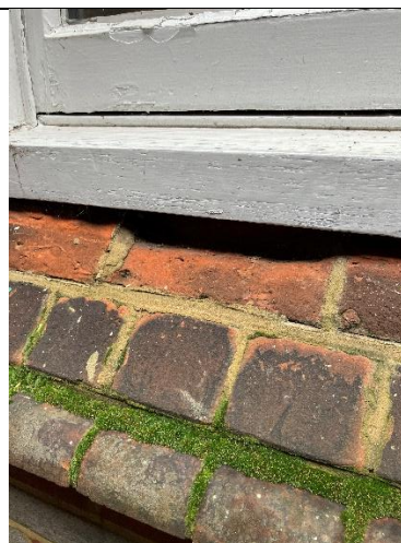
Fig 1.14 – Example of spalled brickwork requiring replacement / repair
