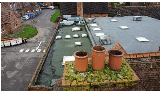
Fig 1.13 – Deteriorated flaunching and pointing to chimney
