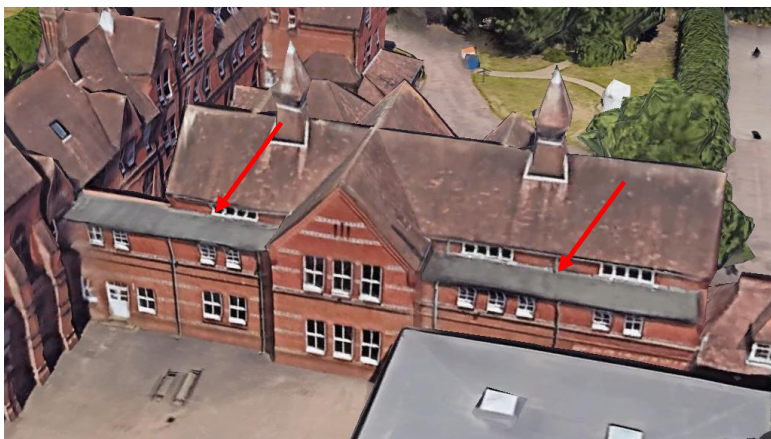
Fig 1.4 – Flat Roofs to be replaced
