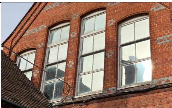
Fig 1.17 – Example of windows in a deteriorating condition
