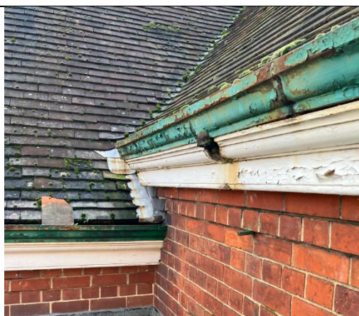
Fig 1.11 – Deteriorated Rainwater Goods
