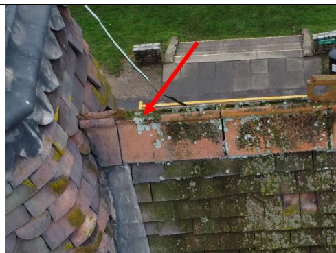
Fig 1.3 – Spalled rolled ridge tile edge
