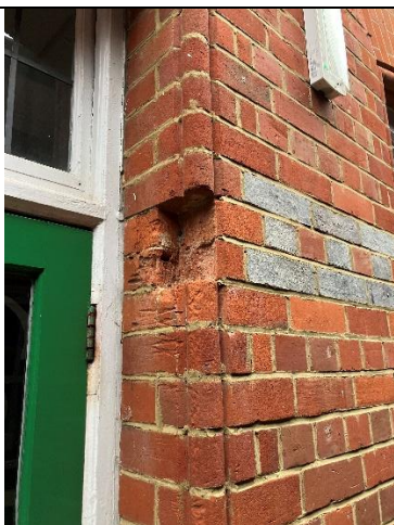
Fig 1.15 – Example of damaged brickwork requiring replacement / repair
