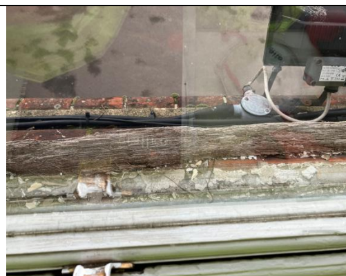
Fig 1.18 – Example of decayed / missing sill requiring replacement
