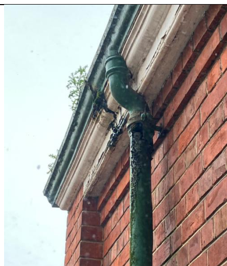
Fig 1.12 – Deteriorated Rainwater Goods
