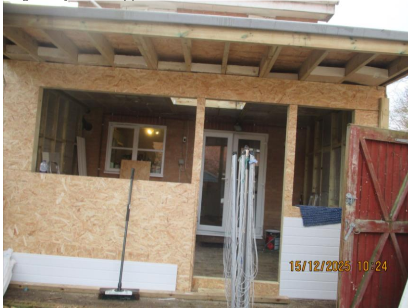
Fig 10: Rear view of 116 Elm Park, provided by Enforcement Team
