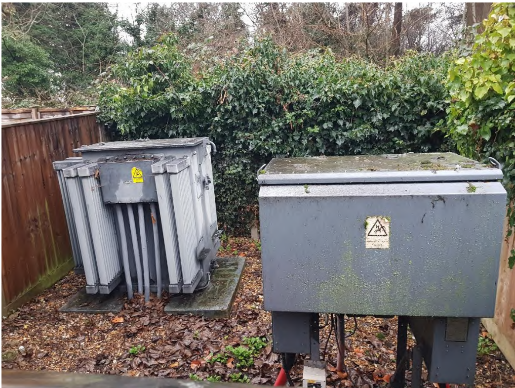
Plate 12: View east showing the small electrical sub-station bounding the site to the north in the north west.
